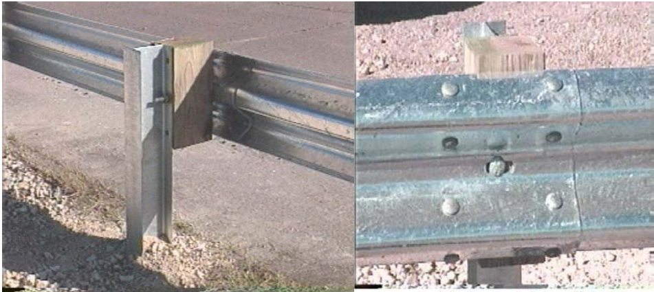
Figure 50. Modified G4(1S) guardrail with routed wood blockouts.
