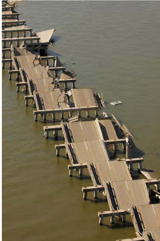
Figure 2-11 Hurricane Damage from Wave Action to Highway 90 in Bay St Louis, MS
