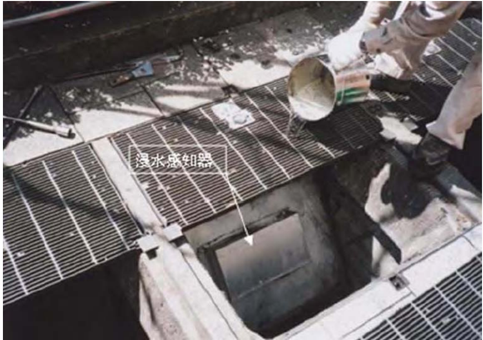
Figure 4-4 Tokyo Metro Ventilation Shaft that can be Closed by Remote Control, Manually Onsite, or Linked to a Flood Sensor
