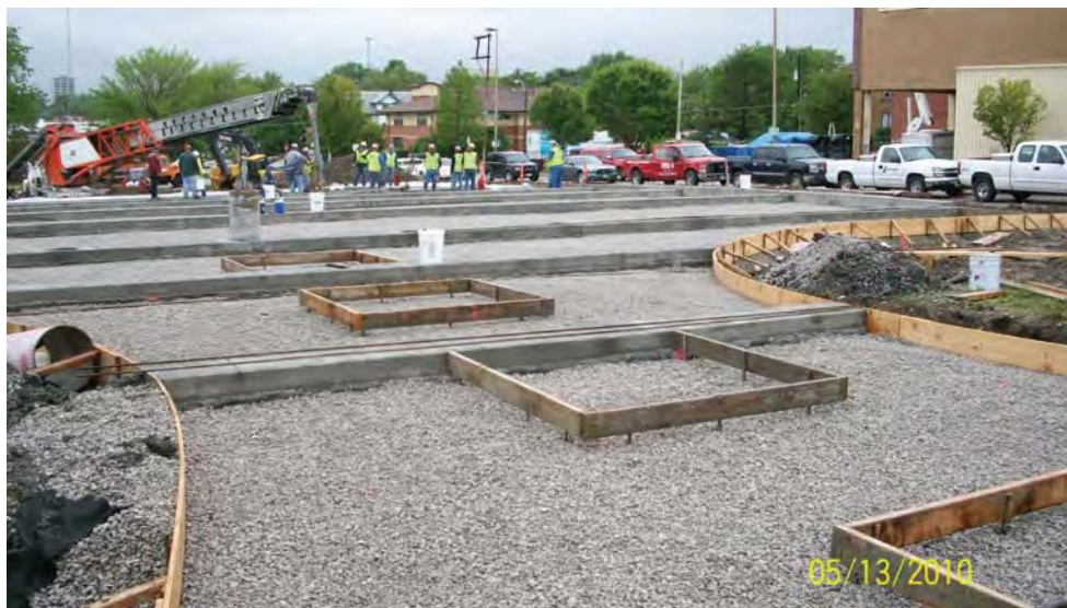
Figure 4-7 Construction of Pervious Concrete Parking Lot that Allows Stormwater to Seep into Ground, Kansas City
