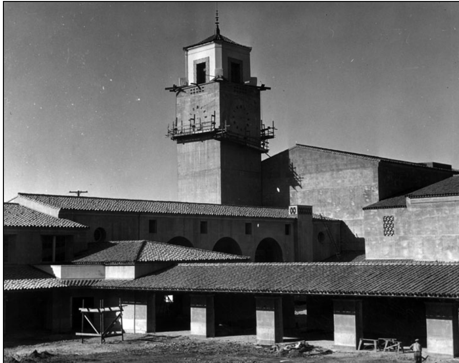
Figure 38 – Union Passenger Terminal under construction, 1938. View is from the taxi area, the south patio is just beyond the covered roof in the foreground. (See figure 41 for plan.) Courtesy of Los Angeles Public Library photo collection.
