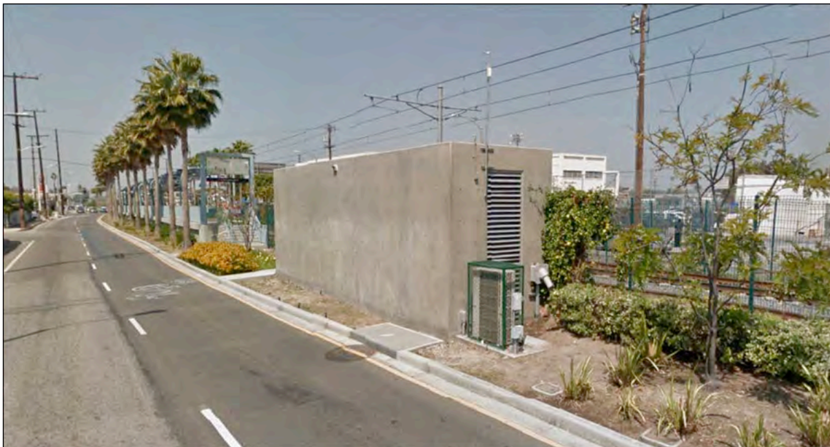
Figure 4.5-16: Example of a Typical TPSS (Traction Power Substation)
