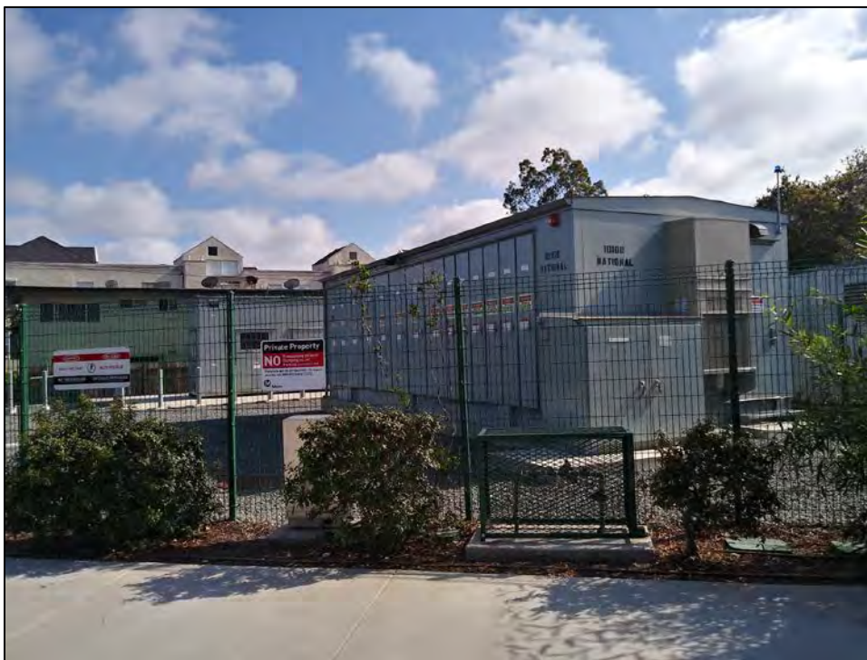
Figure 1-9: Typical TPSS for LRT
