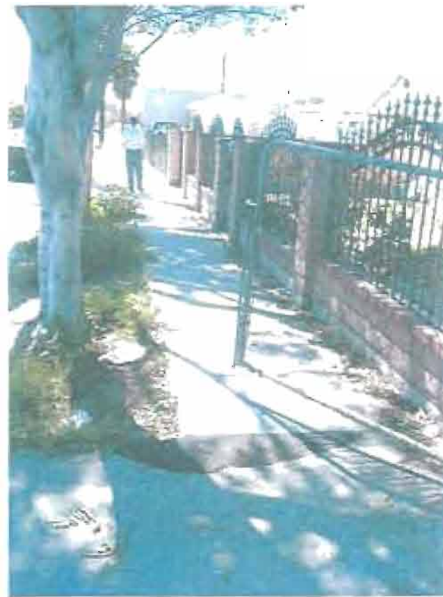
Broken sidewalk on Ford Boulevard near 3rd Street
