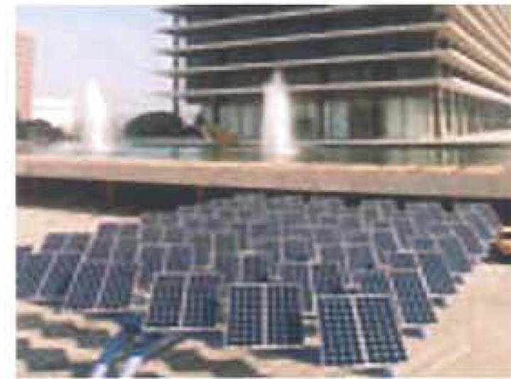
03. Solar panels at LADWP Headquarters
