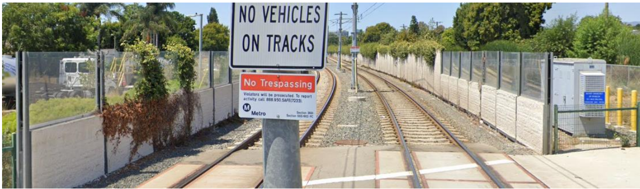
Above are three views of soundwalls adjacent to the existing Metro E Line (Expo).
