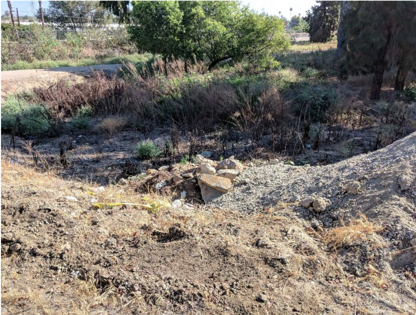
Figure 10 – Southbound off-ramp, north facing view showing existing vegetation and debris
