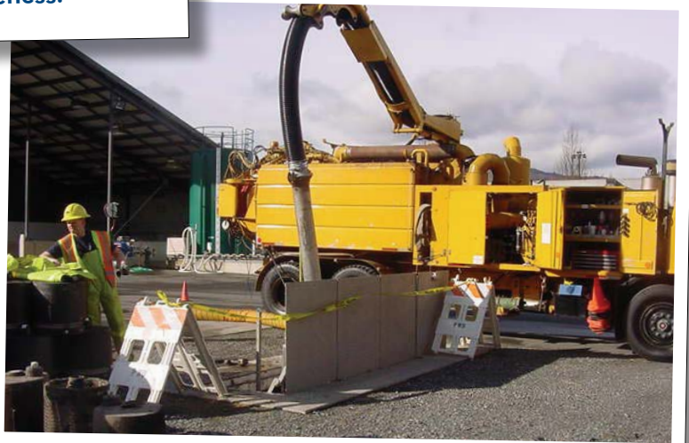
Easy to access treatment system can make a difference in maintenance expenses.
