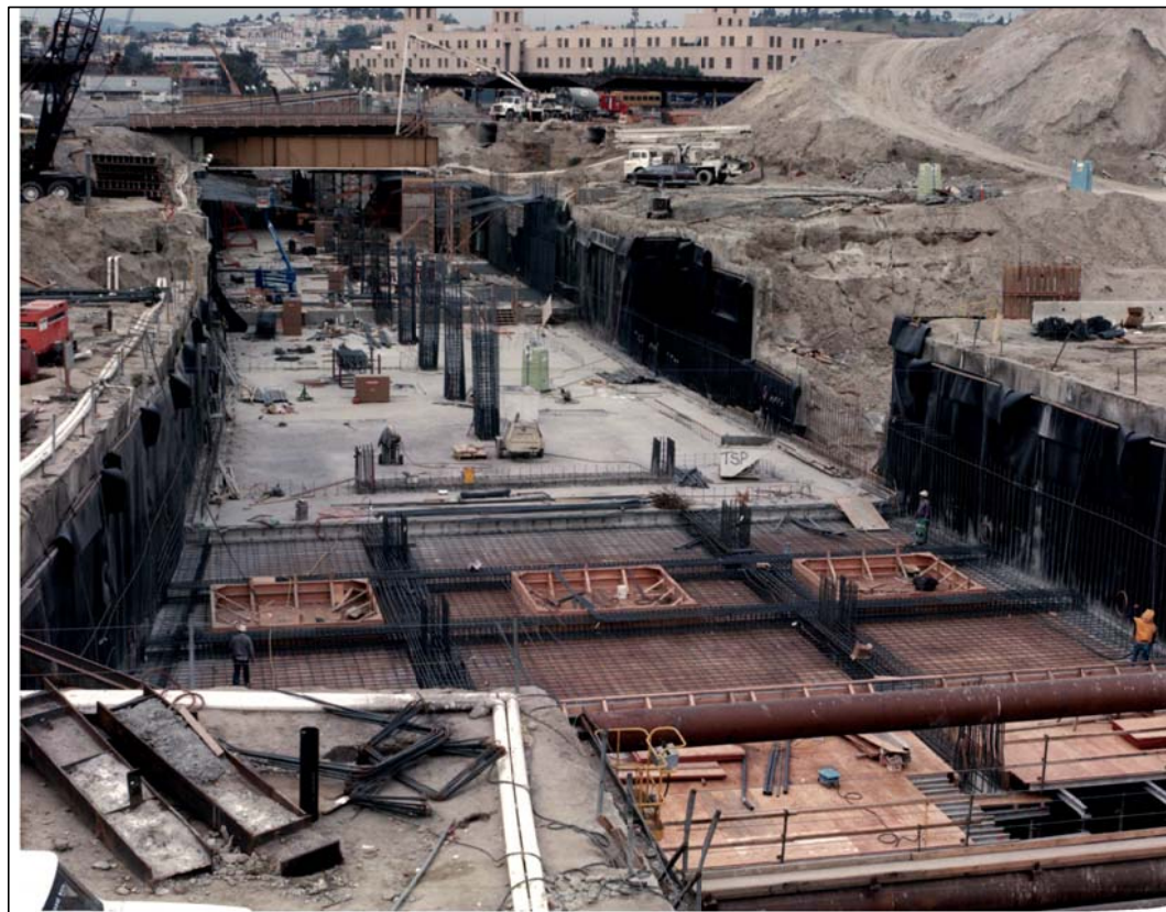
Photo No. 3. Mezzanine floor slab in place with column reinforcement steel protruding. The reinforcement for lift No. 4 of mezzanine floor is being placed in the foreground. Photo Taken: 01/30/90. Source: SCRTRD, 1990a.
