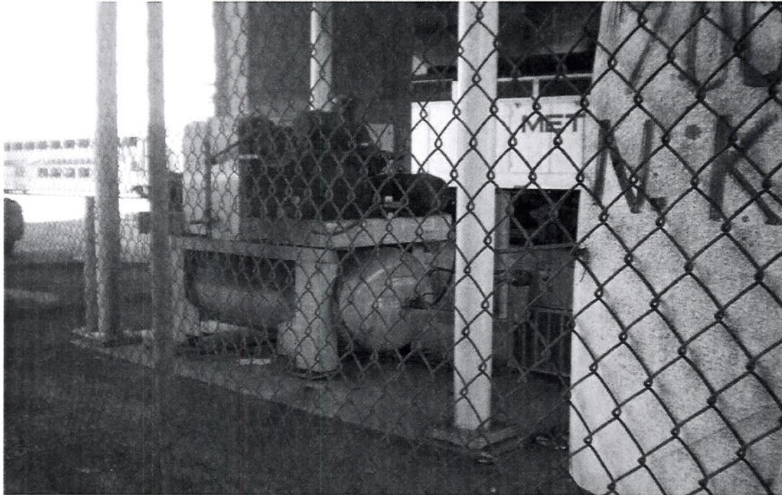
Photo 3 Compressor, south of property
