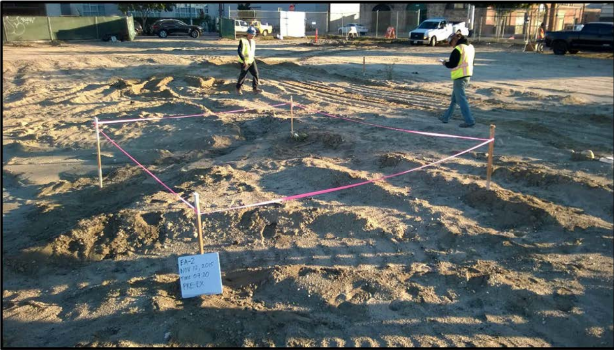
Photograph 5 – View looking north on November 12, 2015 at Excavation Area EA-2 prior to its excavation.
