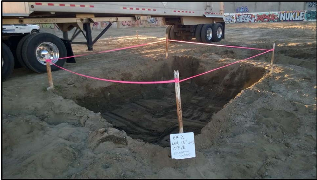
Photograph 17 – View looking southeast on November 13, 2015 at Excavation Area EA-2 after its excavation.
