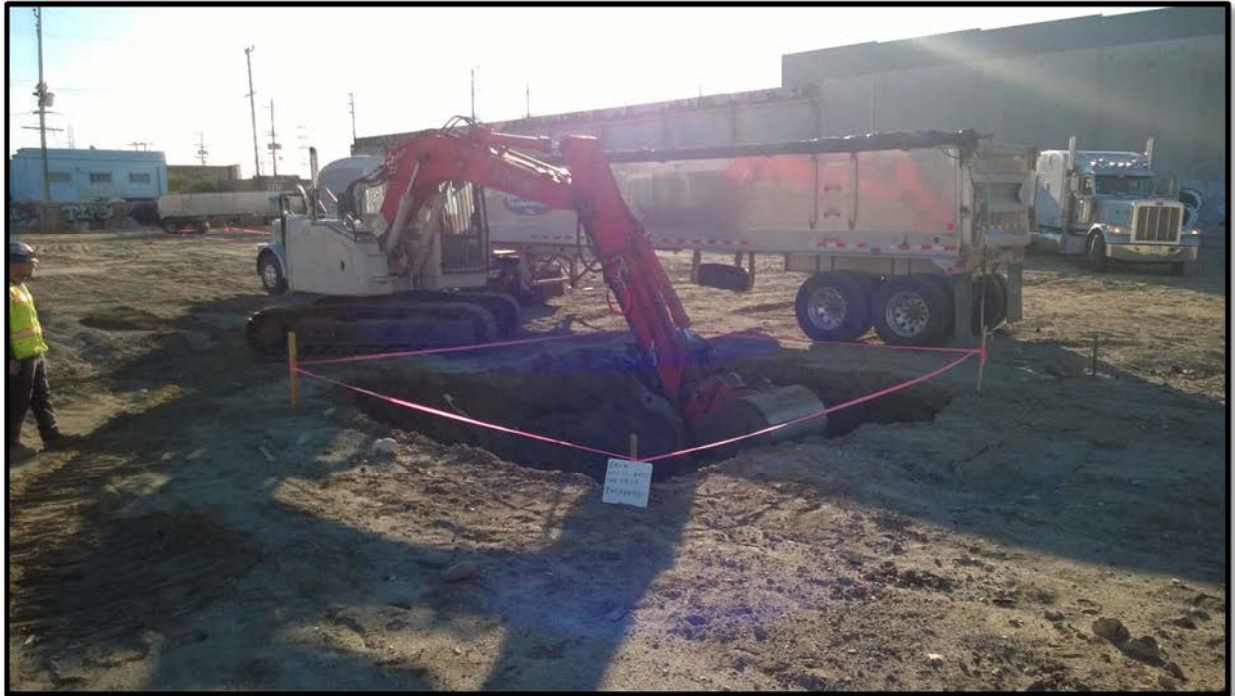
Photograph 9 – View on November 12, 2015 looking southeast at excavation and loading activities at Excavation Area EA-4.
