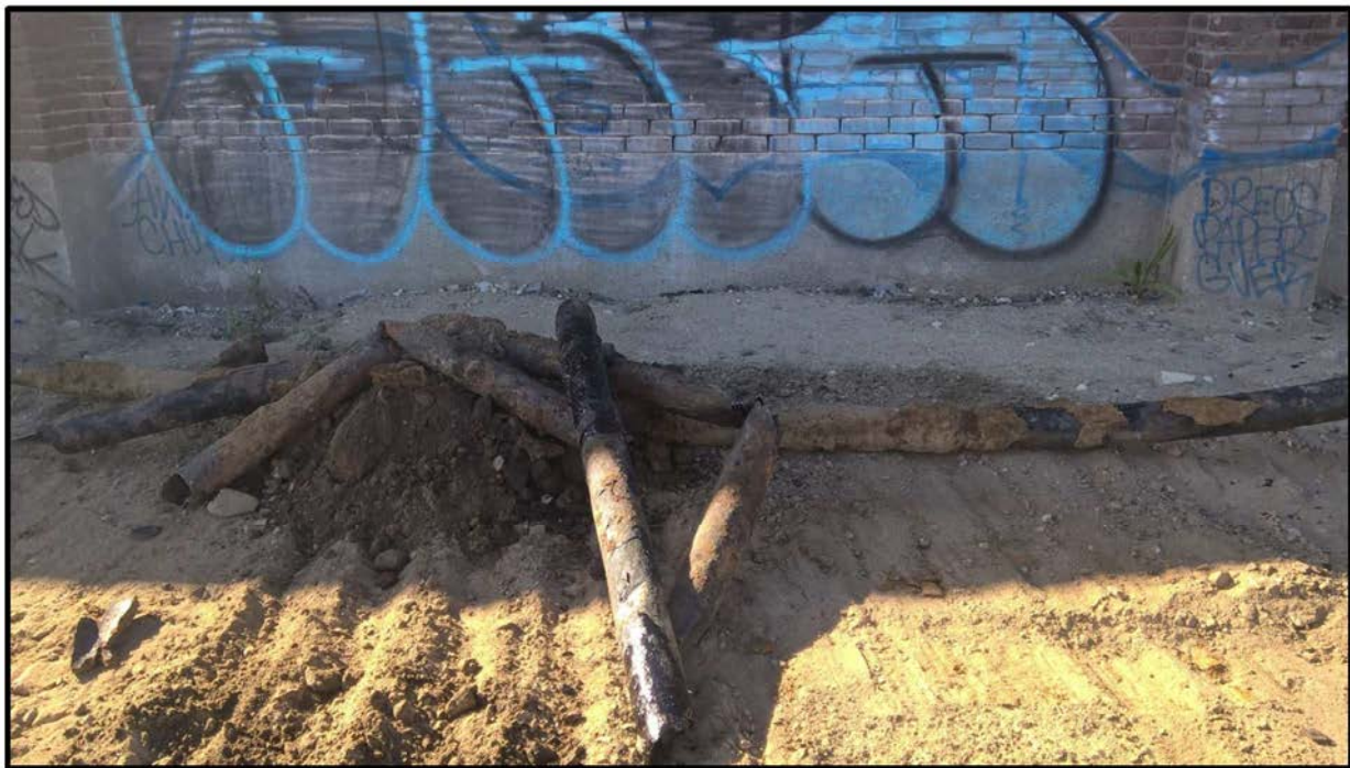
Photograph 20 – View on December 7, 2015 of removed old oil piping and small amount of stockpiled soil before their placement onto plastic sheeting.
