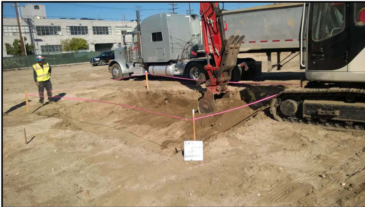
Photograph 14 – View looking northeast on November 12, 2015 at excavation activities at Excavation Area EA-1.
