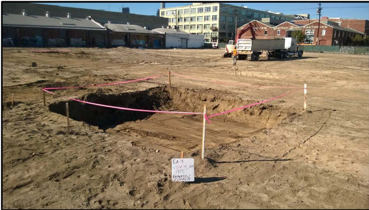
Photograph 12 – View on November 12, 2015 looking northwest at Excavation Area EA-3 after its excavation.
