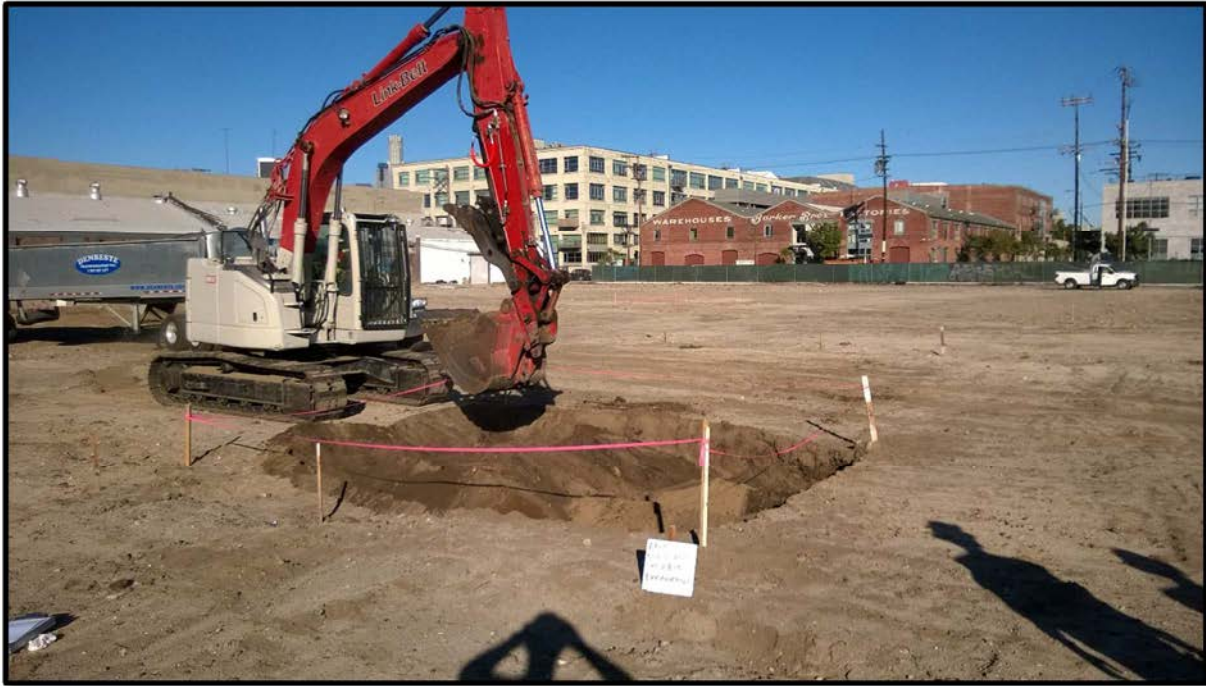
Photograph 11 – View on November 12, 2015 looking north at excavation activities at Excavation Area EA-3.
