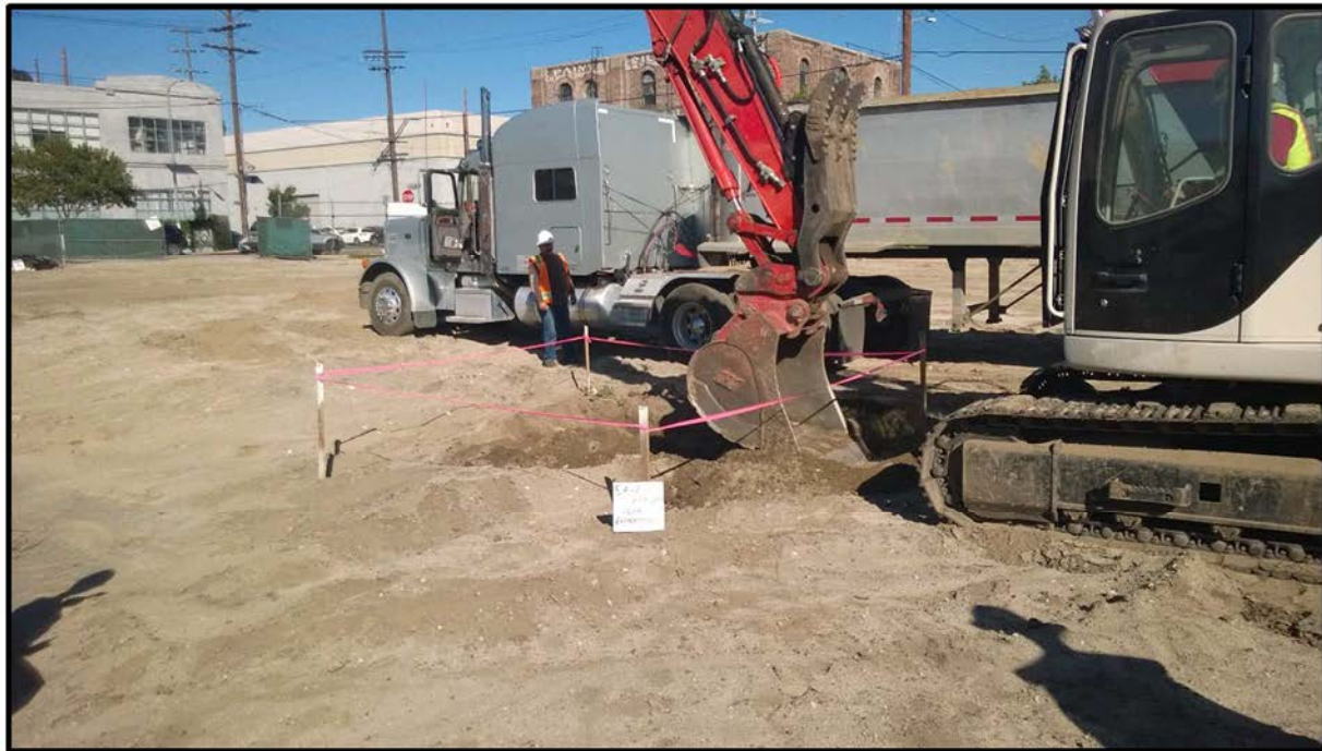
Photograph 16 – View looking northeast on November 12, 2015 of excavation activities at Excavation Area EA-2.
