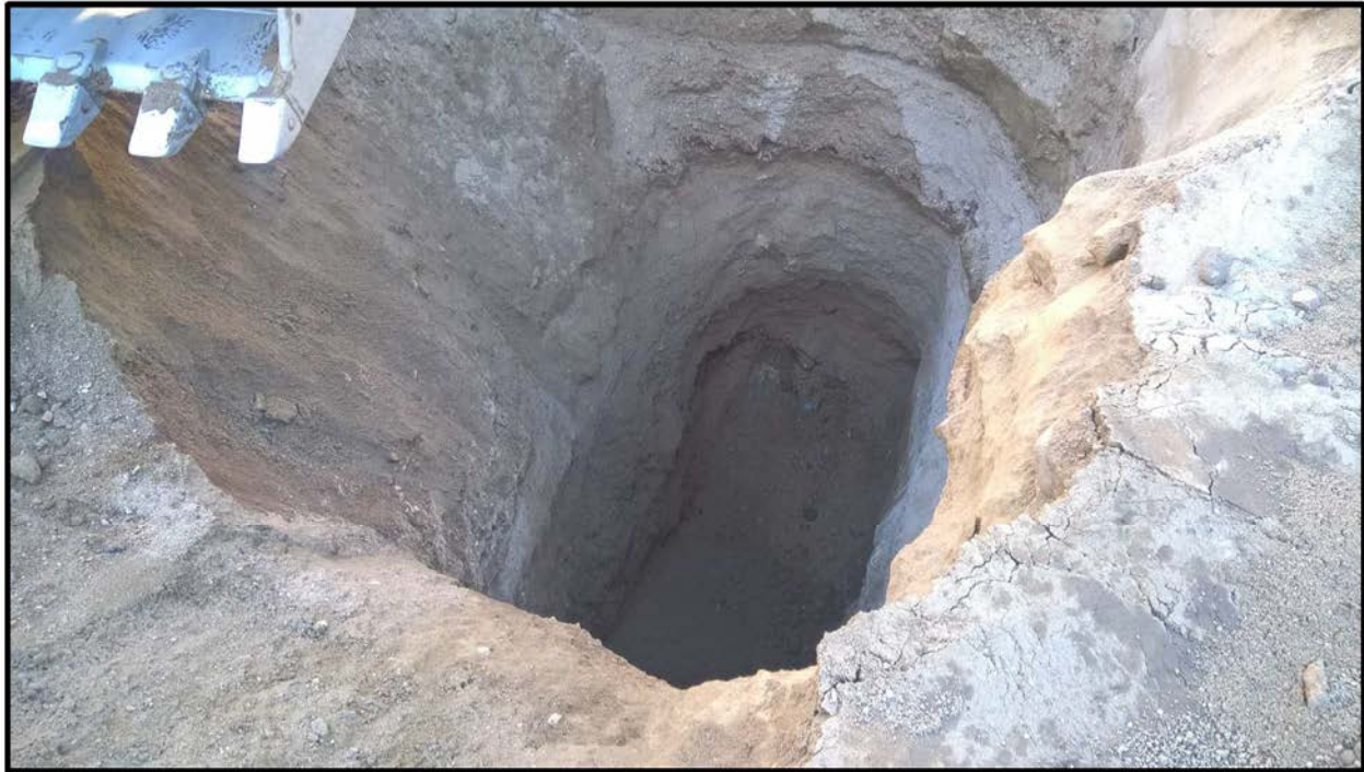
Photograph 28 – View on December 18, 2015 looking at bottom of pothole excavated in floor of Excavation Area EA-5 to approximately 34 feet below ground surface.
