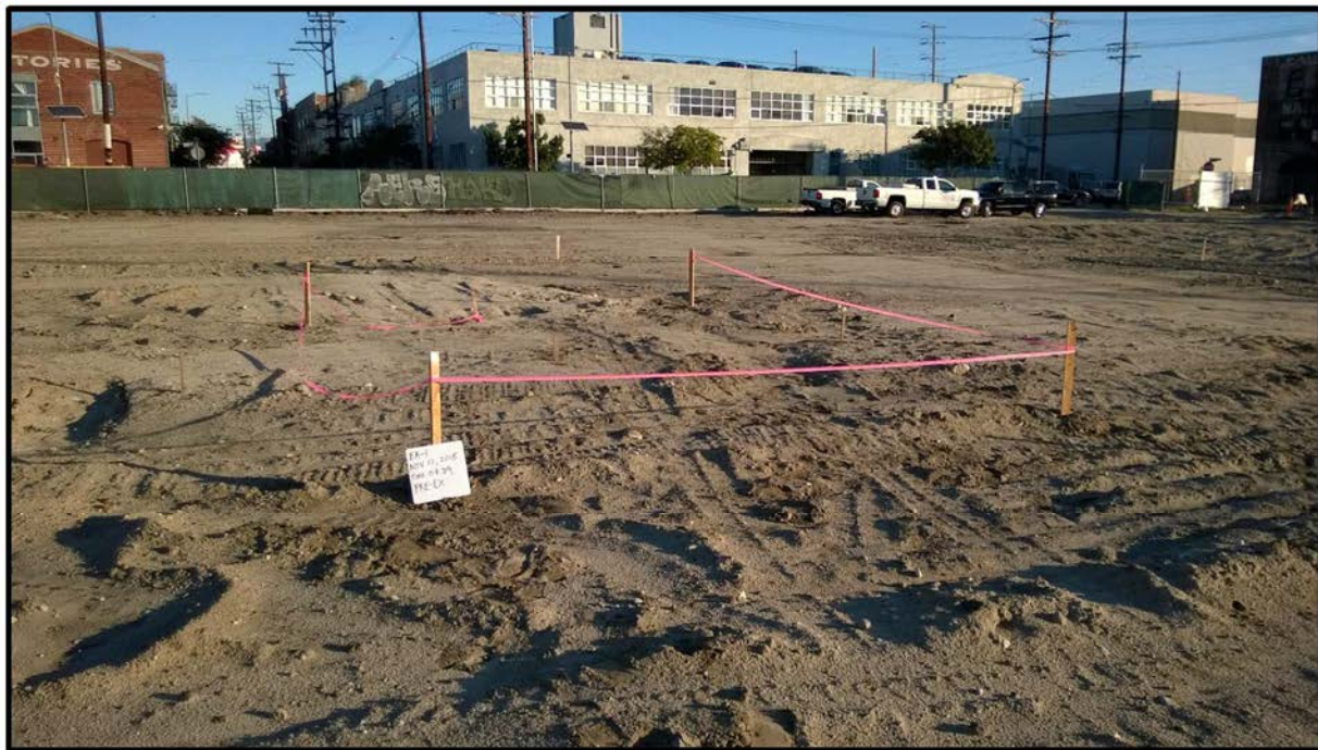
Photograph 8 – View on November 12, 2015 looking north at Excavation Area EA-1 prior to its excavation.
