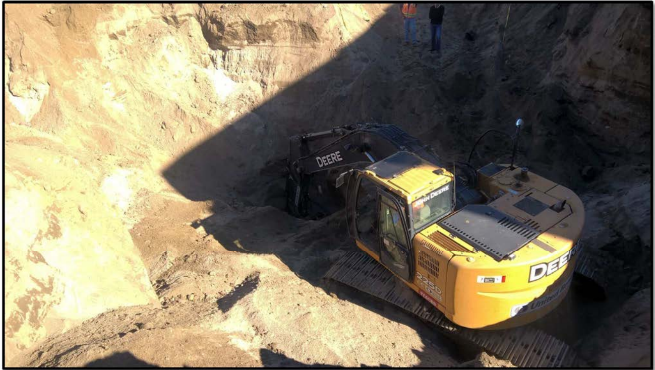
Photograph 27 – View looking northeast on December 18, 2015 of the excavator at the bottom of Excavation Area EA-5.
