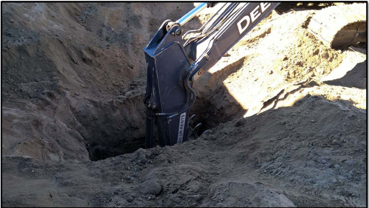
Photograph 30 – View looking west on December 18, 2015 at floor of Excavation Area EA-5 and pothole excavated for collection of post-excavation Sample EA-5-B-61-27.
