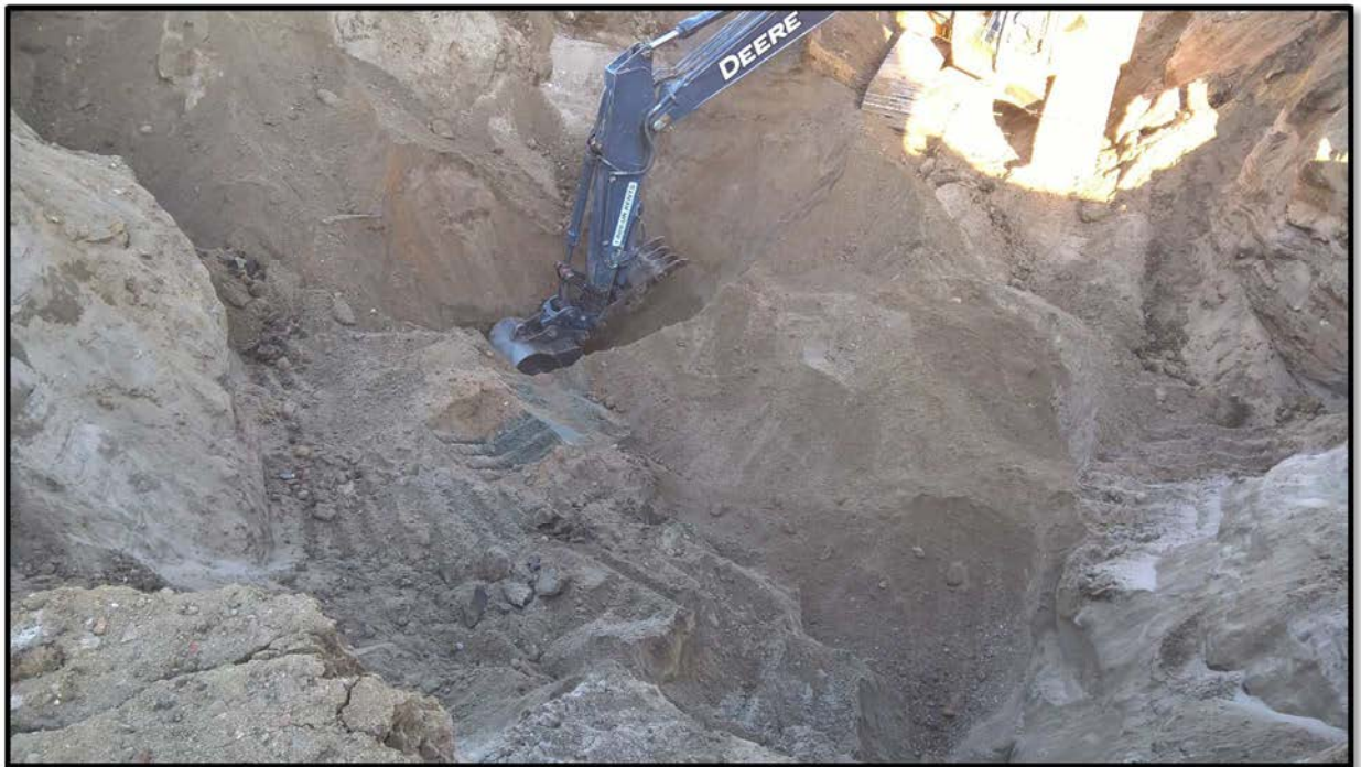
Photograph 26 – View looking north on December 15, 2015 at the bottom of Excavation Area EA-5.
