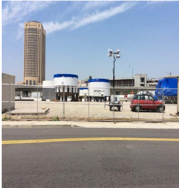
Photo 13: # HDR Map Code # 57 – 510 E. Commercial Street. Site has an open LUST case and is currently used as a construction staging area. The view is toward the north.
