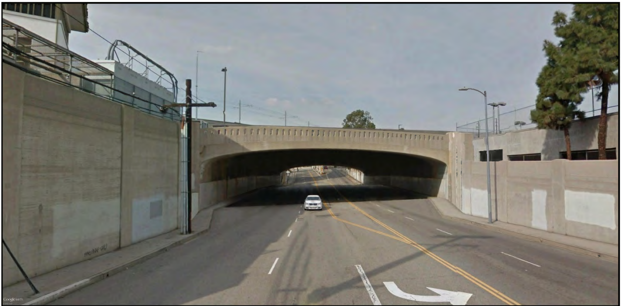
Figure 8-9. Key View #2a – Vignes Street Bridge (view looking west toward bridge) Post-Project Conditions
