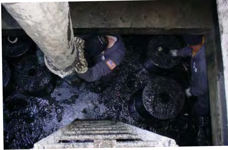
Pollutants must be removed to restore the StormFilter to its full efficiency and effectiveness.
