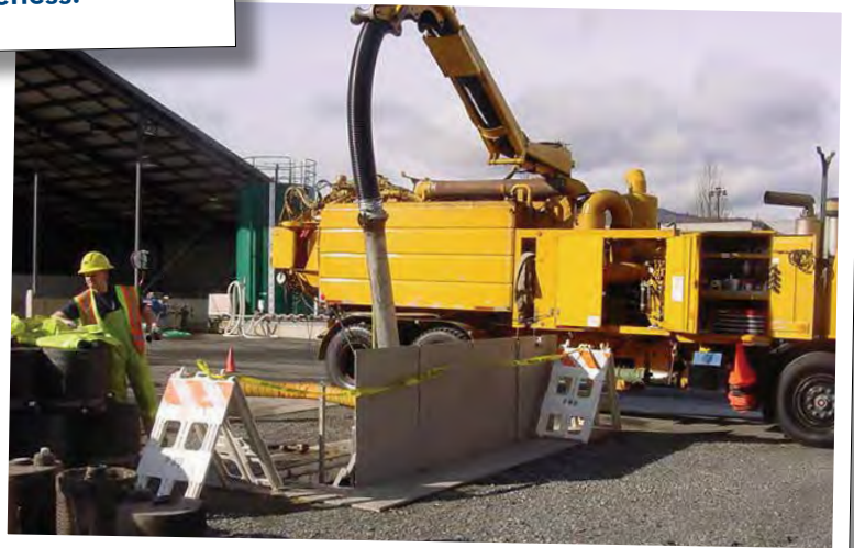
Easy to access treatment system can make a difference in maintenance expenses.
