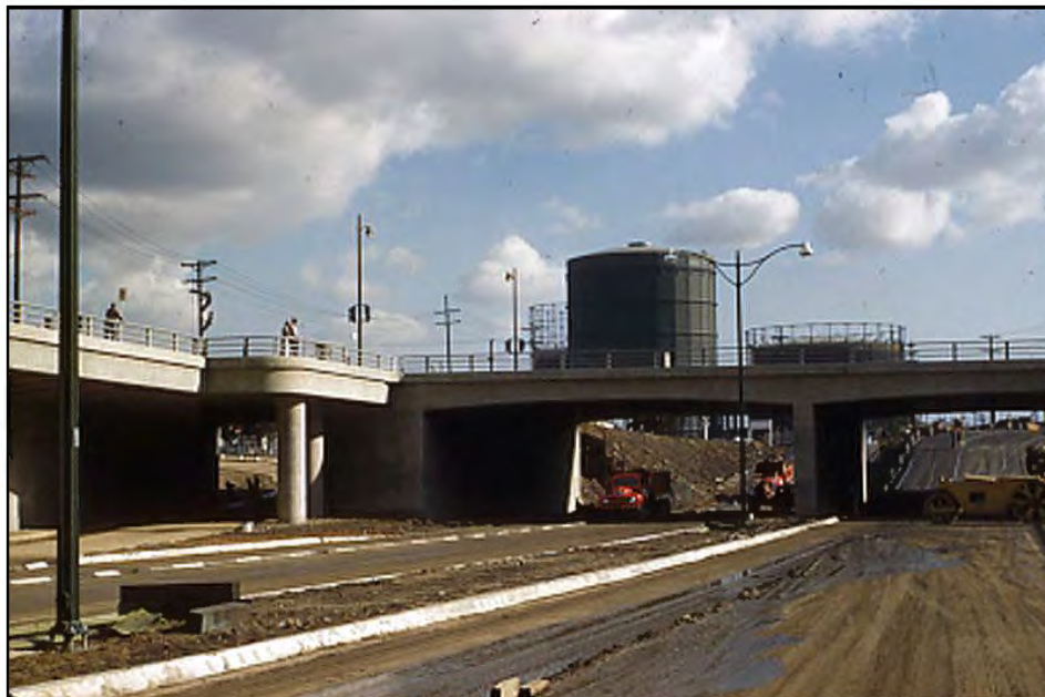
Photograph 10. US 101 Slot under construction, Main and Los Angeles, view to north-east, 1951 (LAPL No. 00109991)
