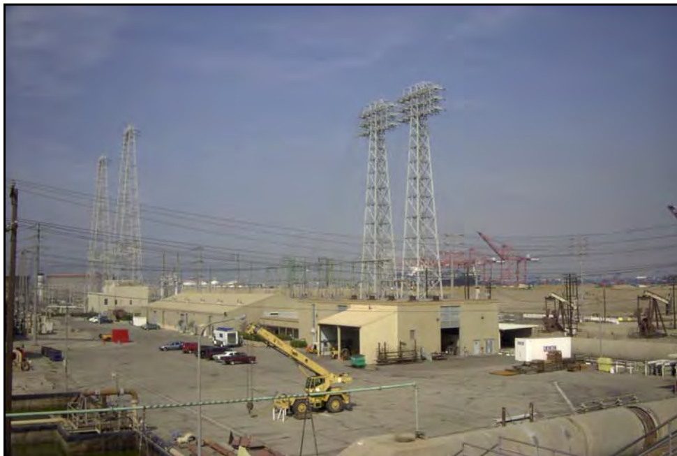
Exhibit 2.1.8-2 Photograph of Transmission Towers
