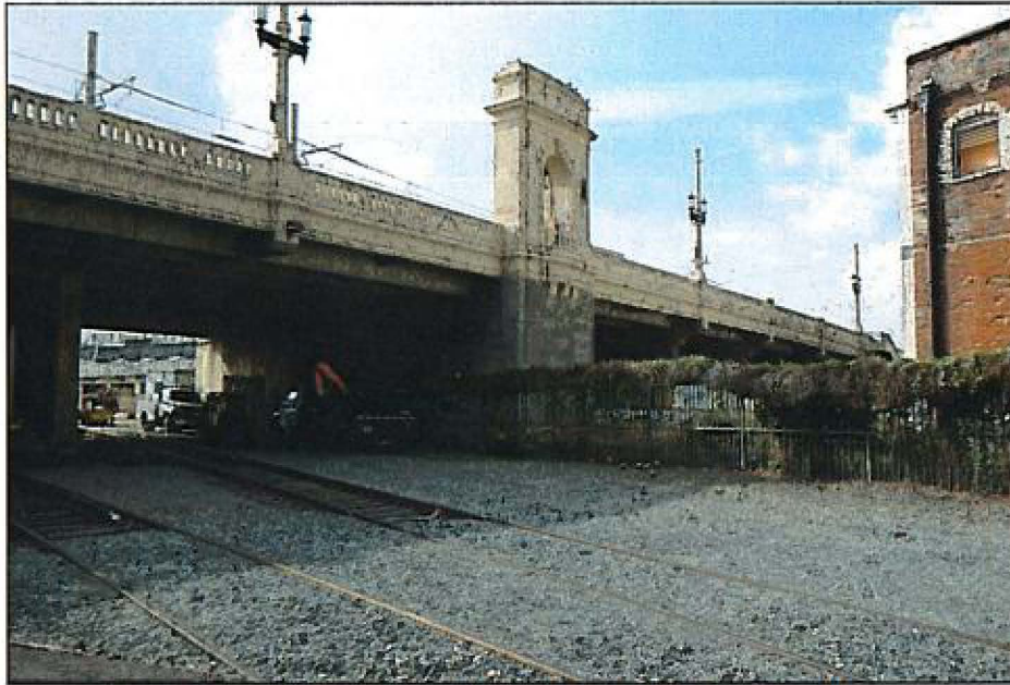
Photograph 2. Widened north side of First Street Bridge over Metro track, view facing southwest, December 6, 2016, IMG_4534
