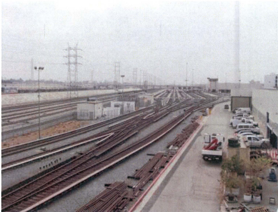
View facing south from 1 st Street at Metro Division 20 Facility. Building 61B is shown right. Railroad tracks and rail yard electrical substation buildings are shown between the railroad tracks (left).
