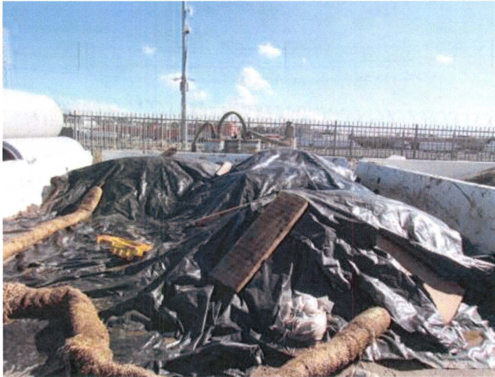
Covered stockpiled soil and gravel stockpile (right) located on the east-central side of the Metro Temporary Storage Yard.
