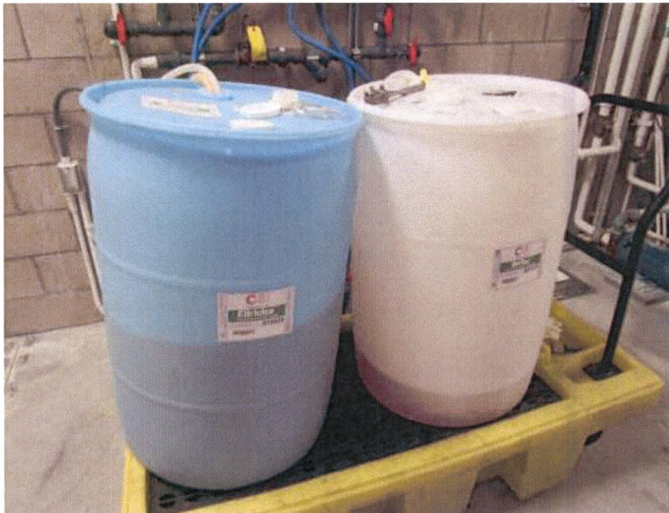
Drums of cleaning soaps located near the softener system inside the Metro Division 20 rail car wash building.
