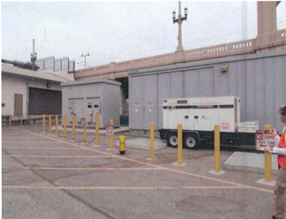
View of transformer station located just south of 1 st Street at the Metro Division 20 Facility.
