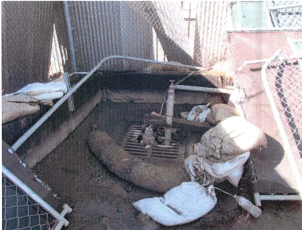
View of a storm drain/sump with pump located on the southwestern corner of the Metro Temporary Storage Yard.
