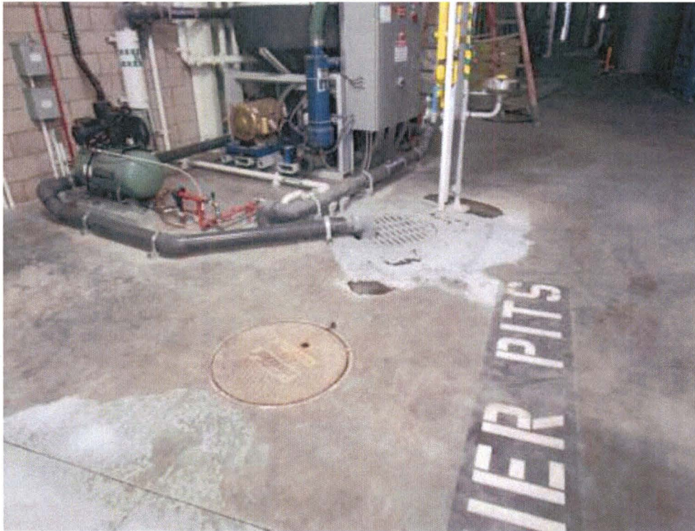
Clarifier pits located inside the Metro Division 20 rail car wash building.
