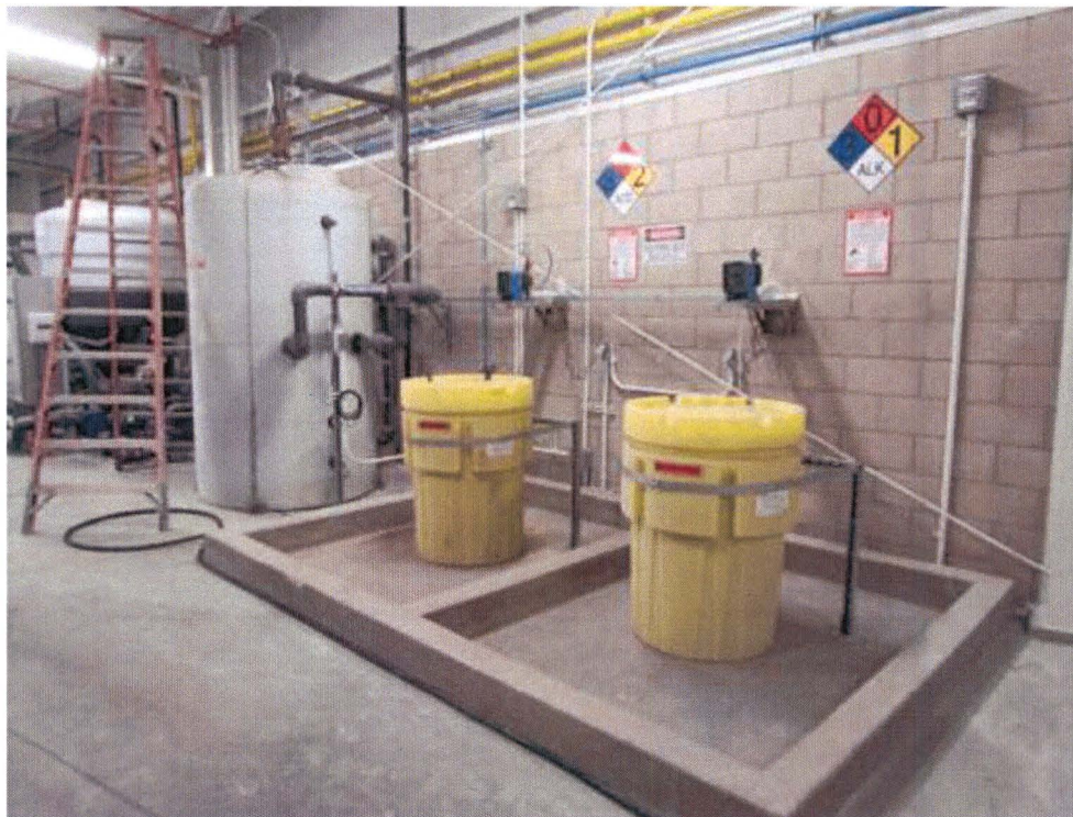
View of caustic soap and sulfuric acid drums, and recirculating aboveground tanks located inside the rail car wash building.
