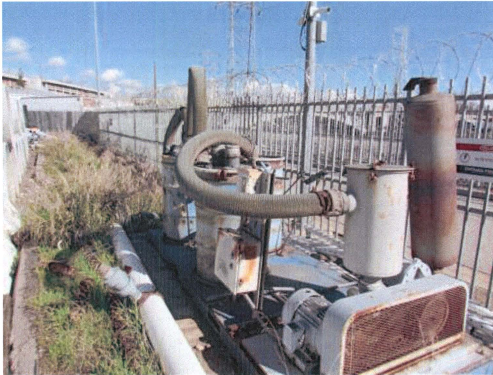
Inactive remediation equipment located on the east-central side of the Metro Temporary Storage Yard.
