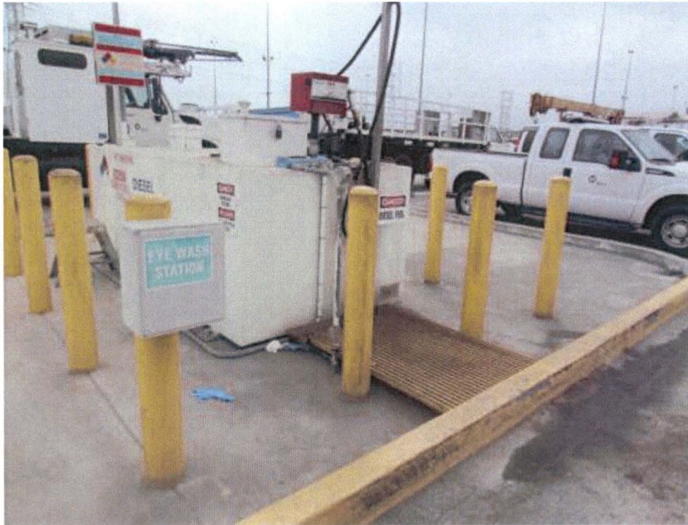
View of 1,000-gallon diesel aboveground storage tank located south of Metro Division 20 Building 61B.
