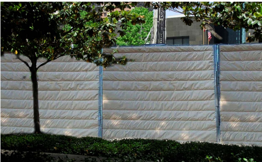
Figure 4.1-7: After View of Flower Street with Construction and Grouting Equipment Facing West Between 5th and 6th Streets
