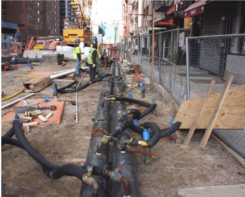
Figure 4-11: Ground Freezing Pipe Installation in New York City, Prior to Starting Freeze
