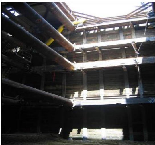
Figure E-3. Typical Soldier Pile and Lagging System (Metro Gold Line Eastside Extension)
