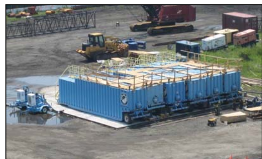
Figure 4-15: Typical Slurry Mixing Plant
