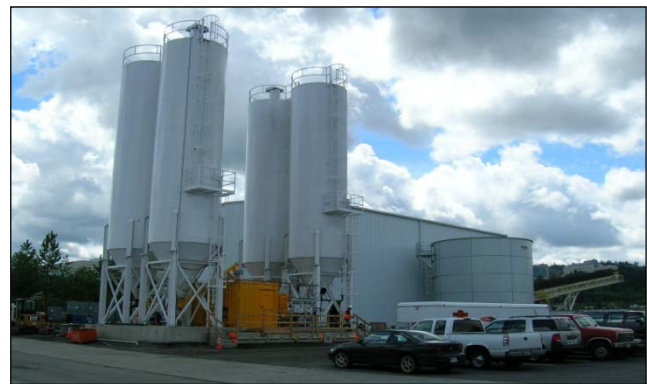
Figure 4-22: Enclosed Slurry Plant with Materials Storage Silos
