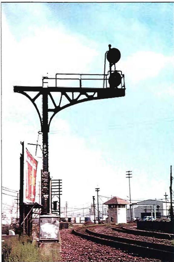
Cantilever signal light controlled from Redondo Junction Tower
