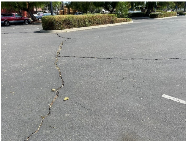
Wider and deeper cracks have a higher potential to enable leaching into the subsurface soil.
