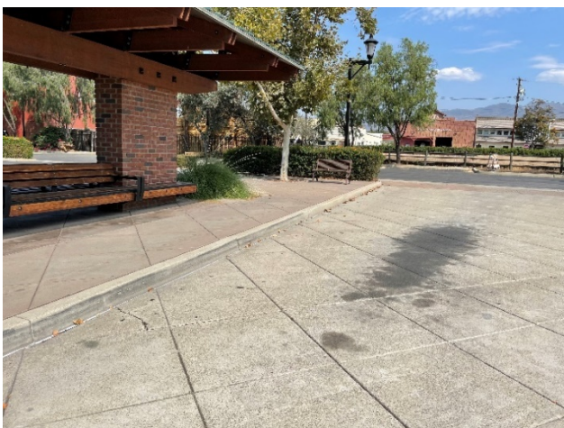
Visible staining was only observed at the center drive aisle of the San Dimas Park & Ride.
