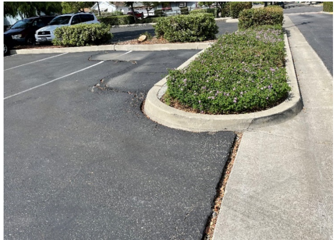
Notable gaps were observed between sections of the asphalt pavement and stormwater drainage route.
