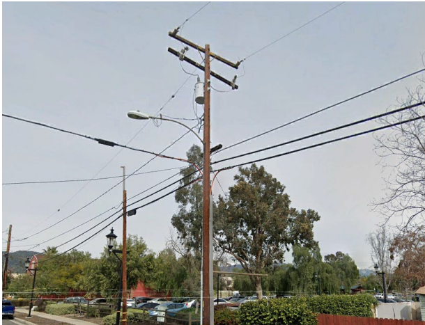
Pole-mounted transformer near the southwest corner of the Subject Property.
