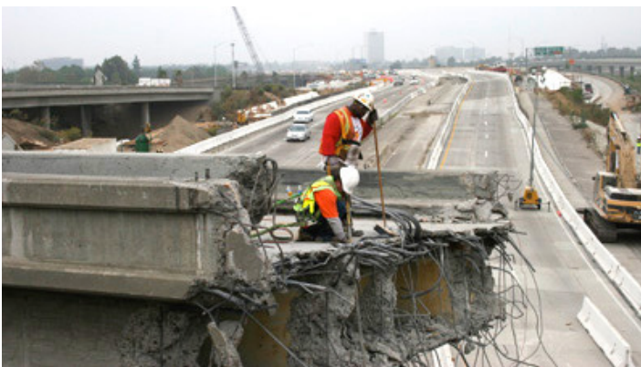
Construction activities can create hazardous waste which will be disposed of at an appropriate disposal facility.
