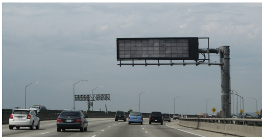
Additional changeable message signs would be added to provide critical information to motorists.
