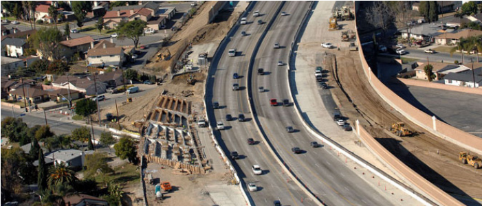
Construction of any of the build alternatives will be a major undertaking. This photo shows a similar freeway widening project on SR-22 in Orange County.
