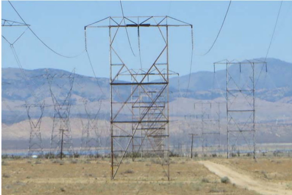
Antelope-Magunden #2 Transmission Line, view towards the north
