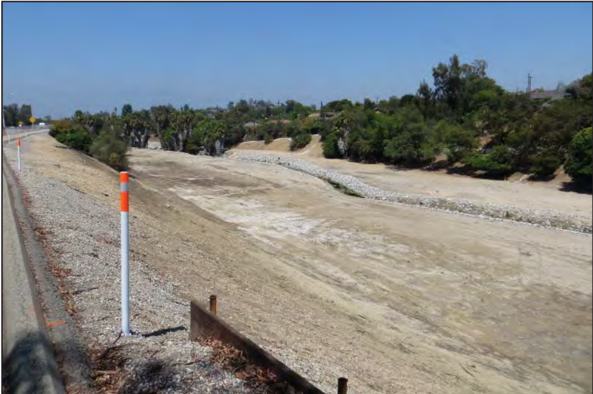
Photo D of Feature 14 Laguna Channel, east of SR 710, north of I 10, facing northeast
