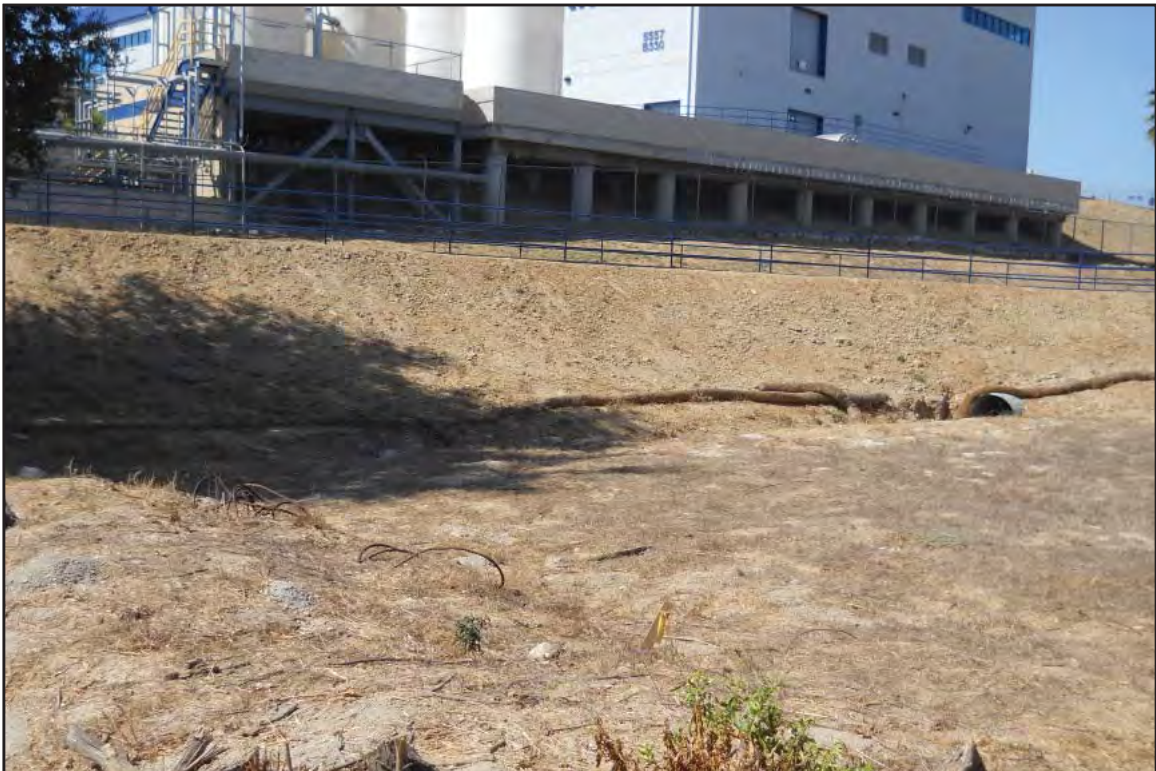
Photo B of Feature 9 Concrete lined ditch near northern SR 710 terminus, facing northwest
