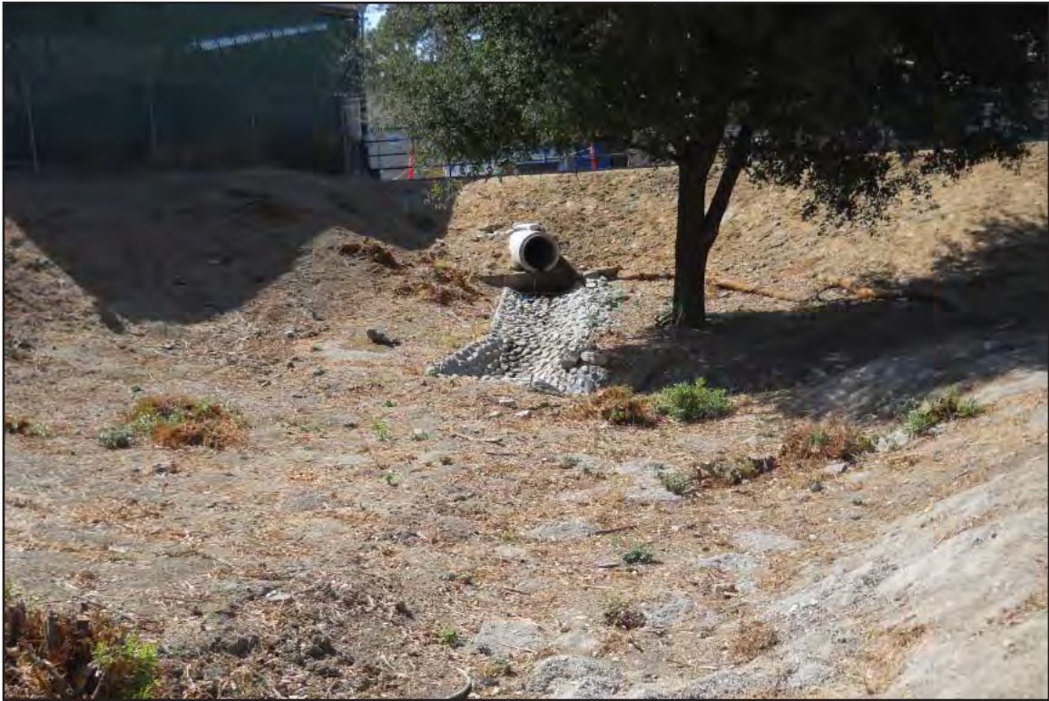
Photo A of Feature 9 Concrete lined ditch near northern SR 710 terminus, facing west
