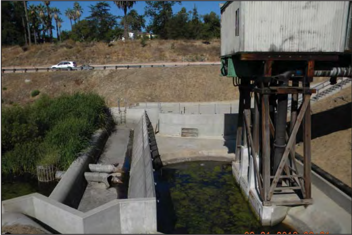
Photo C of Feature 8 Del Mar Pump Station, facing west, photo taken in August
