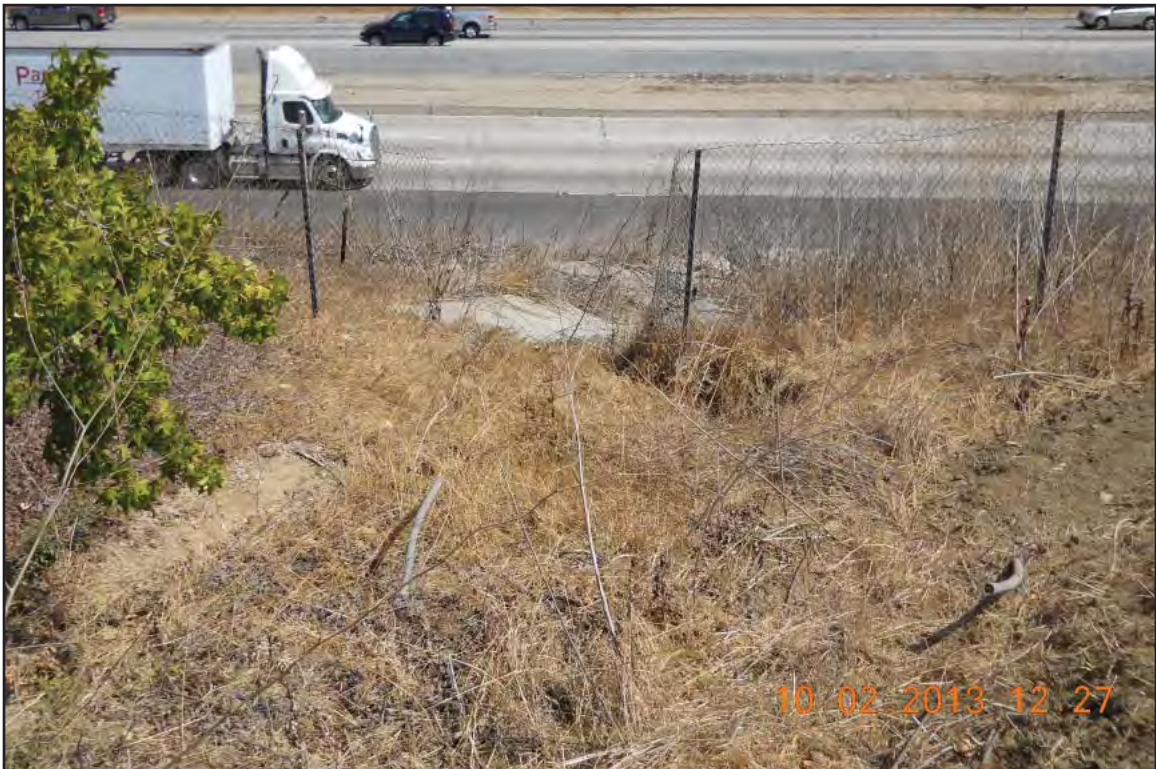
Photo B of Feature 21 Concrete lined ditch west of SR 710 and south of I 10, facing east
