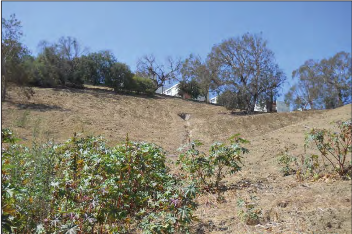
Photo D of Feature 21 Concrete lined ditch west of SR 710 and south of I 10, facing west
