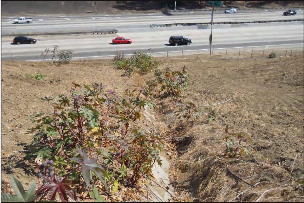
Photo C of Feature 21 Concrete lined ditch west of SR 710 and south of I 10, facing east
