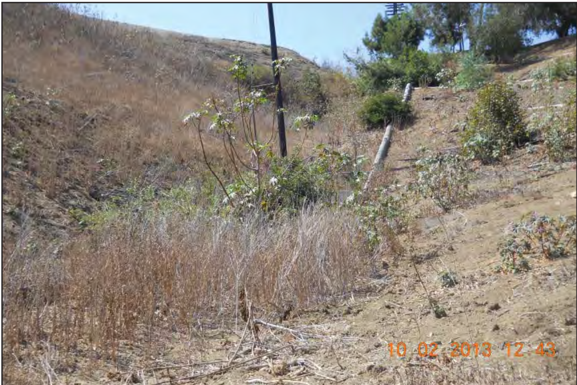
Photo F of Feature 21 Earthen ditch portion, west of SR 710 and south of I 10, facing west
