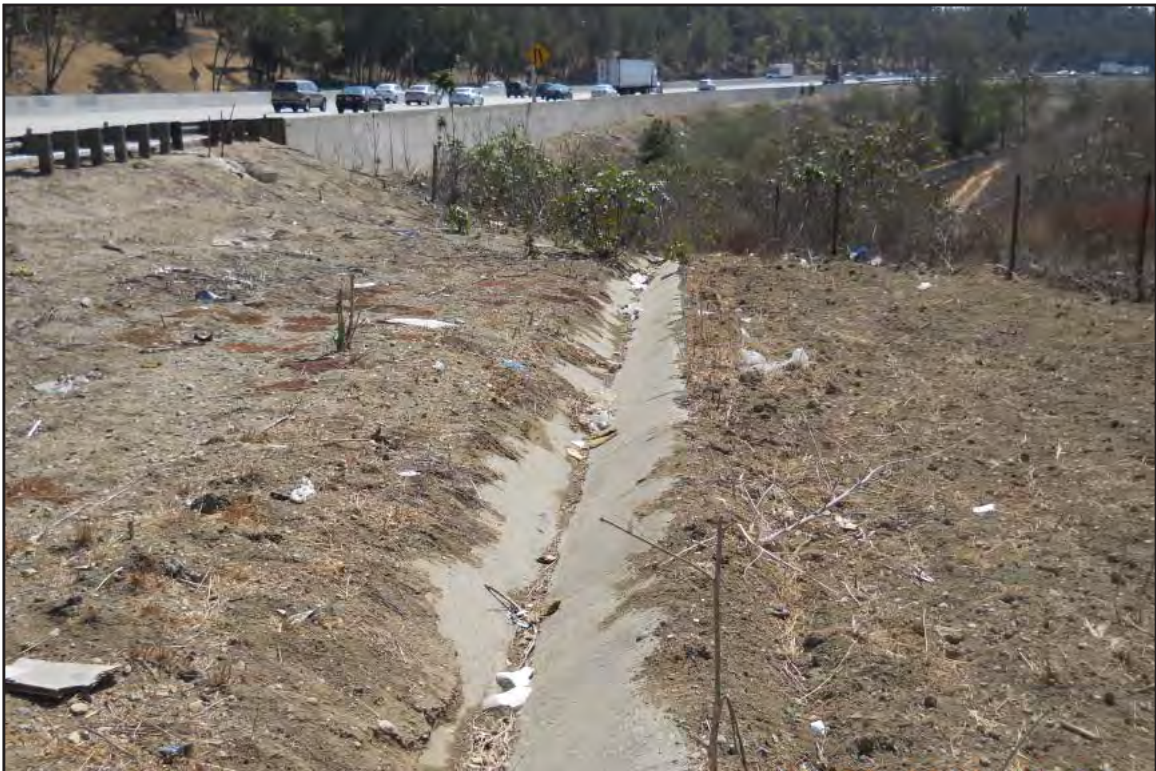
Photo B of Feature 20 Concrete lined ditch west of SR 710 and south of I 10, facing south
