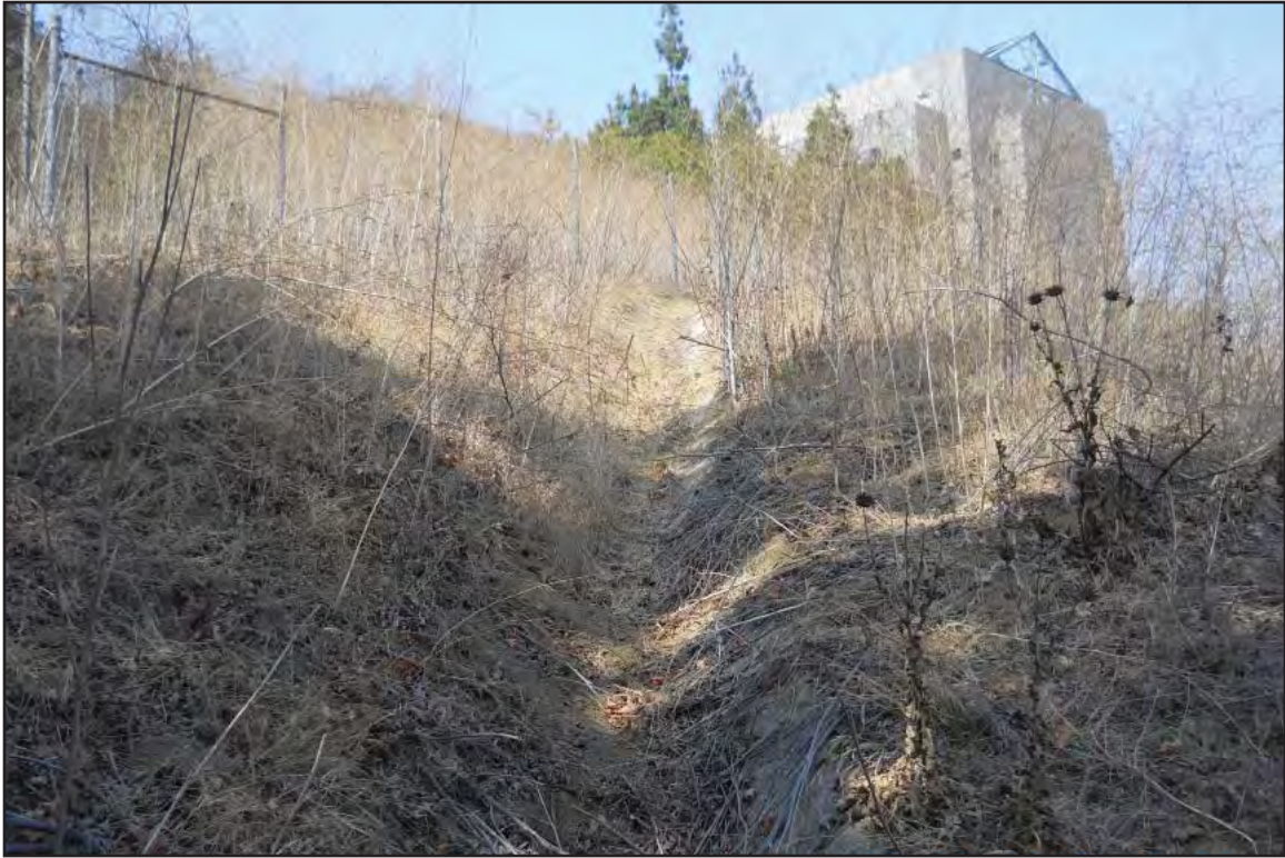
Photo A of Feature 20 Concrete lined ditch west of SR 710 and south of I 10, facing north
