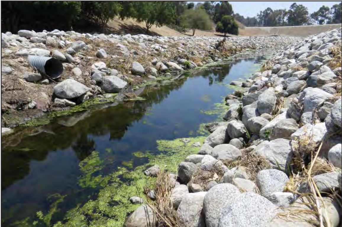
Photo B of Feature 14 Laguna Channel, east of SR 710, north of I 10, facing south
