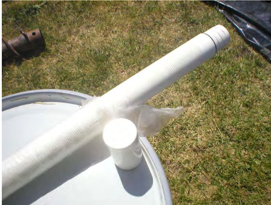
Photograph 9: Close up of the 2-inch SCH80 PVC screened section installed in probe LFG #4.
