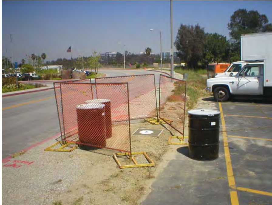
Photograph 4: East-facing view of the completed probe LFG#2. The drums in view were taken to a central collection point for characterization and disposal.
