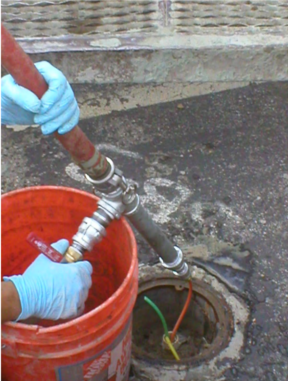
Photograph 15: View of typical probe abandonment system. The valve system was attached to the drilling rig pressure pump; the tube to the old probe was attached than grout was placed until it would not accept any more. The top of the probe was drilled out to 5 feet bgs and backfilled with bentonite. The surface was capped with concrete.
