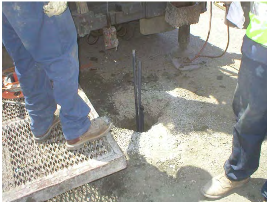
Photograph 5: A typical probe completion prior to the installation of the wellhead. This is the completed probe LFG #3. The probe casings are arranged with the deepest probe to the north and the shallowest probe to the south.
