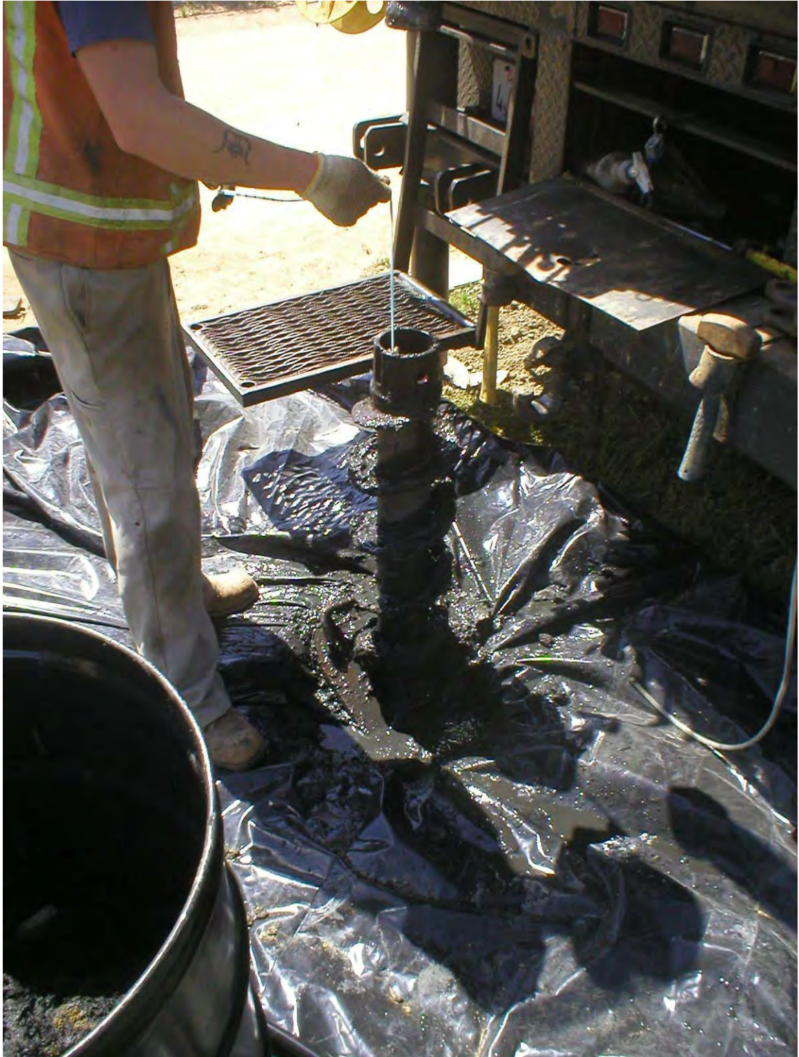
Photograph 8: Close-up of refuse encountered in probe LFG #4. Material was black and saturated with a very strong LFG odor.
