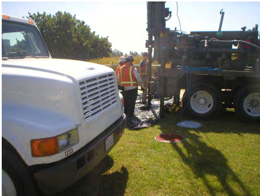
Photograph 7: Drilling activities for probe LFG #4. This probe is located near the site's helopad.
