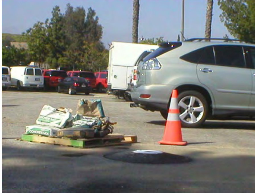
Photograph 6: Completed views of probe LFG #3. Note that the wellhead has been set high—this is at the request of the client. This parking lot is scheduled to have approximately 2 inches of asphalt added as a repaving project.
