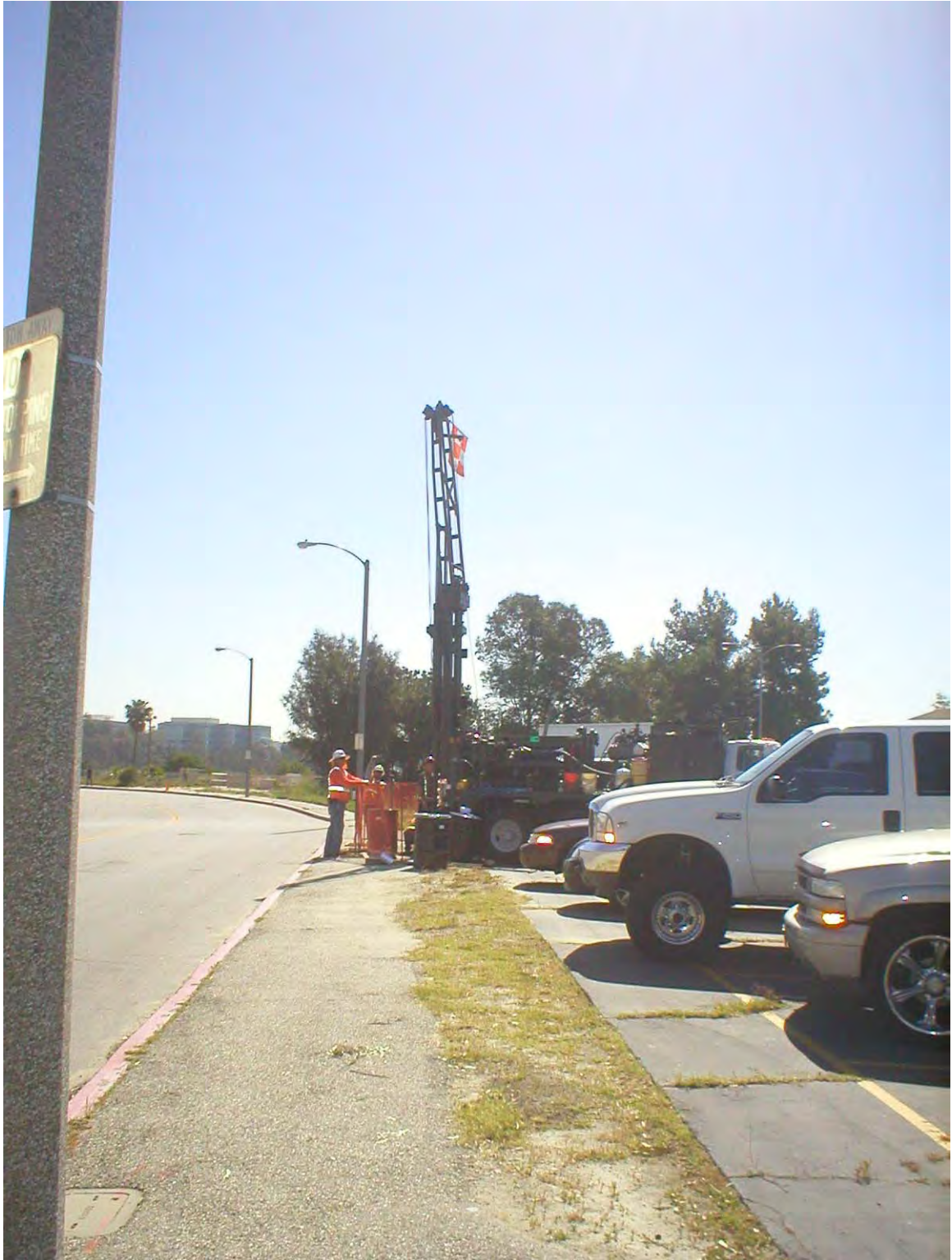
Photograph 3: Drilling and setting probe LFG #2. The probe was completed in the green belt between Sheriff Road (left) and the parking lot (right).
