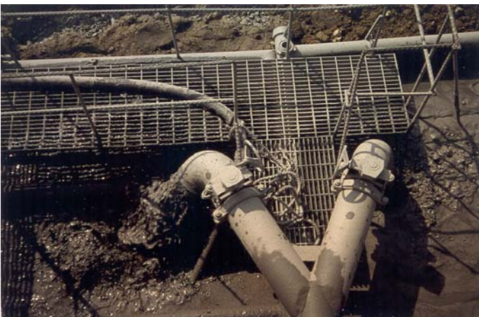
Slurry pumped from tunnel entering separation plant
