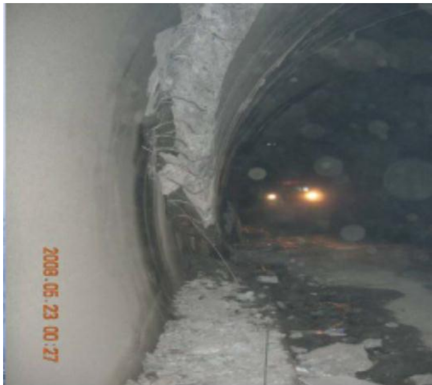
Figure 4. Shear Damage to Section of Longxi Highway Tunnel in China, Subject to about 1 m Fault Offset, following the 2008 Wenchuan Earthquake (Li, 2012)
