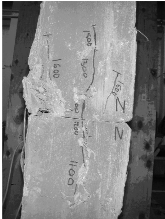
Figure 10. Segment Testing Showing Tensile Splitting Cracks Originating at the Segment to Segment Contact (Swartz et al., 2002)
