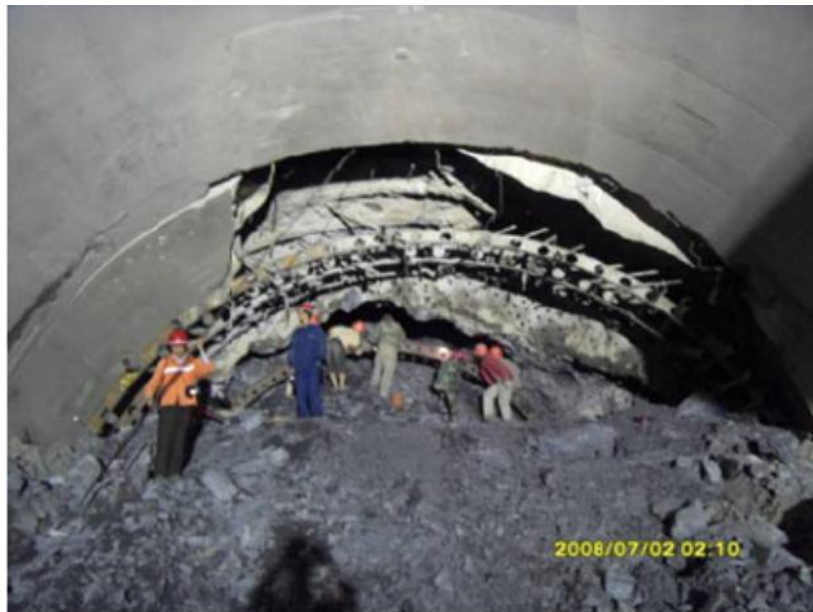
Figure 5. Collapsed Section of the Longxi Tunnel, China following the 2008 Wenchuan Earthquake (Li, 2012)
