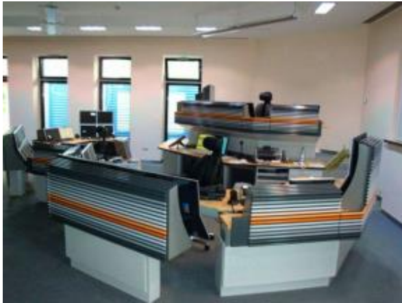
Figure 3 Operator and Supervisor Workstations
