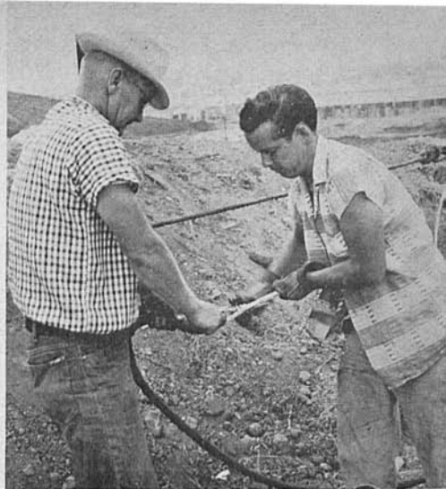
FASTENING CABLE TO ROPE are Messrs. Hornseth and Planellas. Power winch on truck located east of Boyle will then pull rope, cable, into place.
