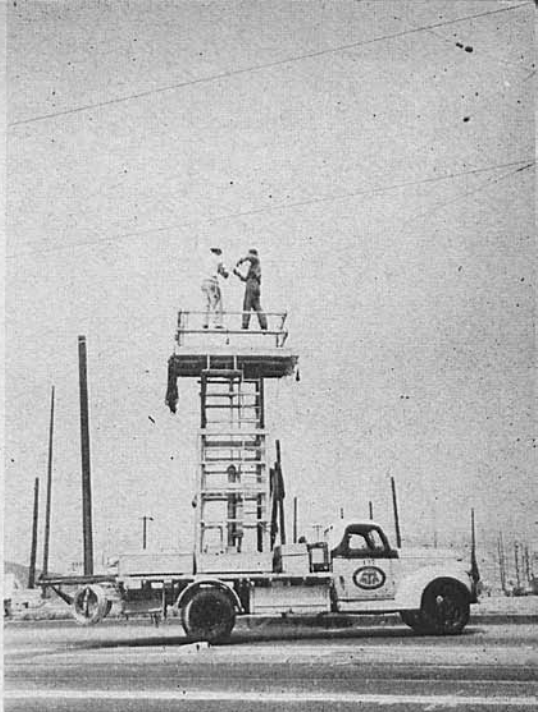
ON TOWER TRUCK, Linemen Harold Jones, left, and Joe Carter string guy wires under 2500 lbs. tension as support for trolley wire, which is pulled into curved shape over detour at 2800 lbs.
