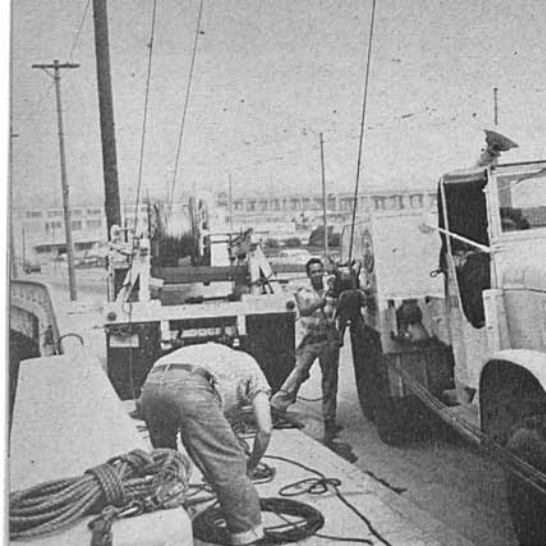
AT POWER WINCH on truck located on 7th St. west of Boyle are Heavy Gang Foreman B. C. Hornseth, left, and Lineman Joe Planellas, threading rope over crossarms of poles on 7th.
