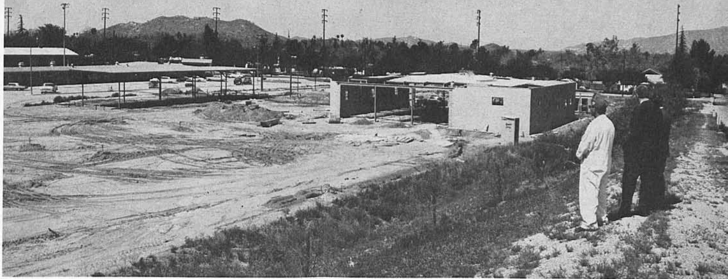
PROGRESS on the new Riverside Garage as of Apr. 14 is viewed by, from left, Riverside Mechanic Otis C. Balthrope, Chief Engineer Ernest R. Gerlach, and Senior Transportation Engineer David D. Canning. Buildings beyond cars are not part of MTA property. View is of rear of buildings, looking from the east.
