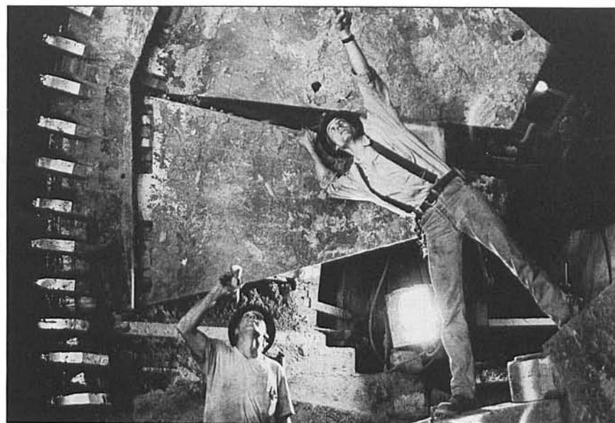
Tunnel crew members inspect the shield of a tunnel machine. The circular shield is about 22 feet in diameter.
