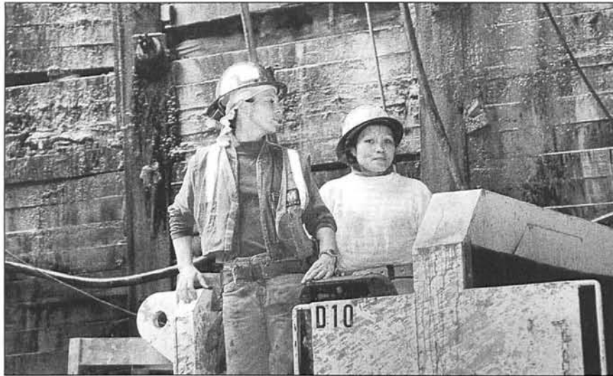
Eve Reeves (L.) prepares to dismount from a tunnel locomotive, a "loci," driven by co-worker Celsa Rijos. The women are members of the mining crew constructing Metro Red Line tunnels beneath the Santa Monica Mountains to link Hollywood and North Hollywood. (Photo by Tracey Mostovoy, The Perfect Exposure.)
