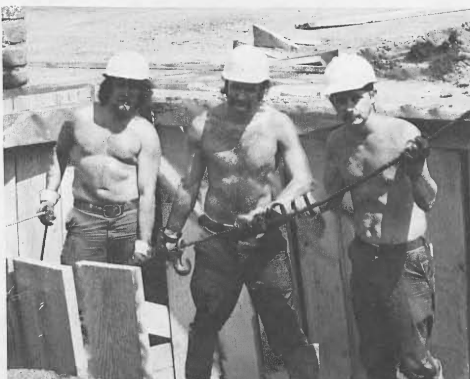
Looking up from installing a fuel tank at Division 7 are three members of the building and grounds section. From left are John Markles and Richard Kovach, both Laborers "A"; and Warren Hulbert, Maintainer "B".
