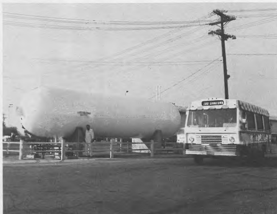
A BIG TANK FOR THE MINI BUSES—An 18,000 gallon propane fuel tank was recently installed at Division 3-10 to fuel RTD's growing fleet of mini buses.
