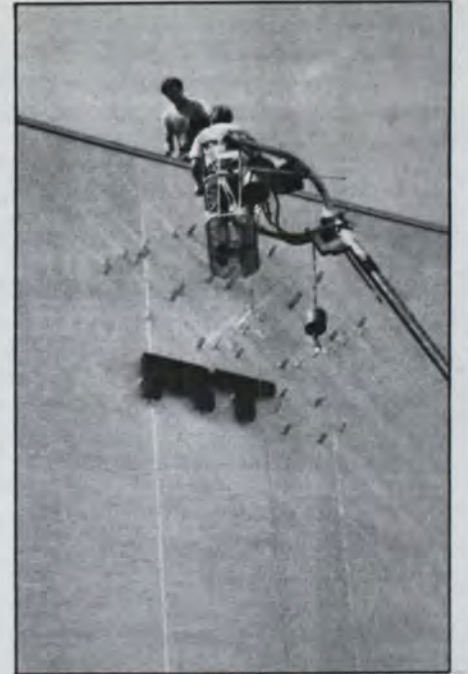
Slowly does it as the worker in the crow's nest is handed off the letters from his cohort on the roof.
