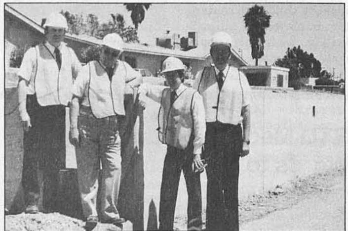
At the future site of Wardlow Station, Richard Morton, George Cowley, Art Peterson, and Ed Vandeventer examine the foundation for the station platform.
