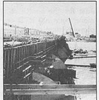
A view of the falsework and forms used to cast the concrete foundation of the new rail bridge spanning the Los Angeles River for the Long Beach - Los Angeles Transit Project.
