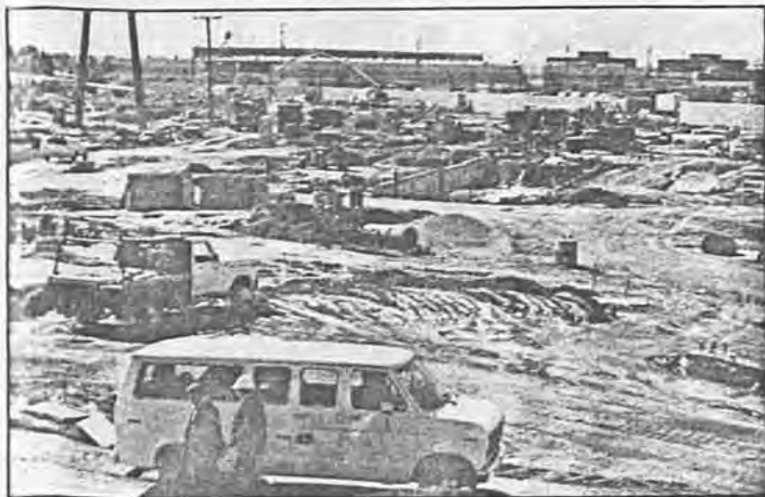
Division 11 for the Light Rail system is now under construction. The site is located along the Long Beach Freeway, near the Del Amo exit. The foundations for the Operations Building are shown in the background in the photo on the left. In the photo on the right, a view of the north end of the
