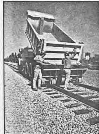
The rock or ballast is shoveled from this holding truck which has special wheels to ride the rails.
