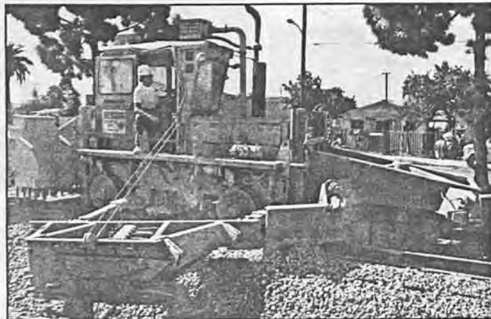
This equipment driven on the track spreads ballast (the rock which supports the track) on the line between Rosecrans and Imperial.
