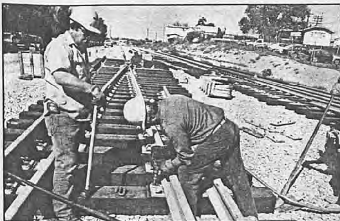
These workers install the first rail on the Long Beach-Los Angeles Line at the Willow Street pocket track.
