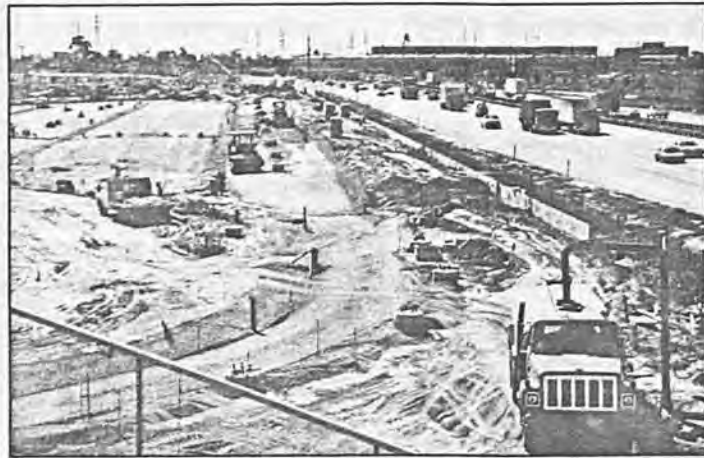
Division 11 storage yard. The loop at the end of the yard is visible. The division will have storage and maintenance capacity for 80 vehicles; and, initially will service the 54-vehicle Long Beach-Los Angeles and Century rail transit project fleet.
