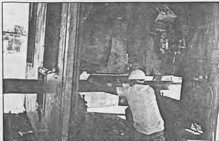
A worker welds the lengths of rail to form a quarter-mile long section of rail. This welded rail will reduce the noise level as the rail car travels along the track.
