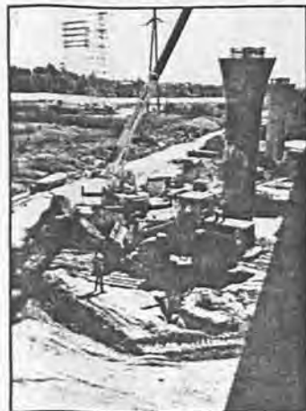
A bridge column under construction near Division 11. This column will support the main line bridge over the Union Pacific line and the Long Beach Freeway.
