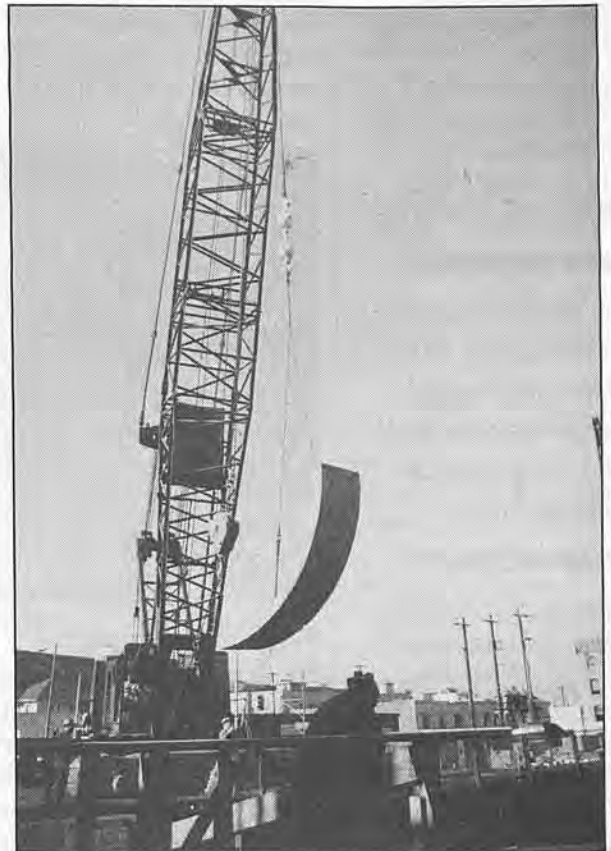
Concrete liner ring segments are hoisted by crane and then lowered into the 80-foot deep excavation shaft to be used at the primary liner for the tunnel that is now being carved by the digger machine.
