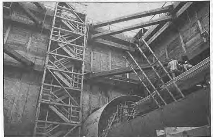
The tunnel boring machine advances through the earth cutting out a circumference through which will fit a subway.
