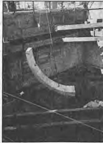
The liner ring segment is lowered into the hole where it will be put into place and bolted together creating a tunnel opening of 22 feet in diameter.
