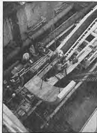
Workers below await the liner ring segment so that they may position it in the space in the tunnel formed by a shield which pushes ever deeper into the earth. The workers wait atop the conveyer section of the tunnel boring machine which carries the muck dug off and spills it into muck wagons.
