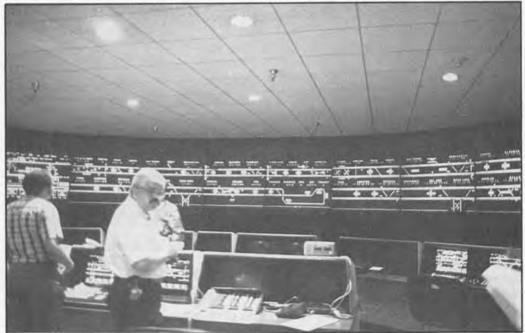
TOS Jess Diaz looks up from his computer screen to check an alarm signal indicating crossing signals were down at Vernon Station.
