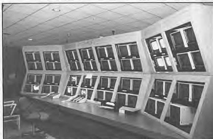
Sixty-two closed-circuit televisions will allow observers to surveil activity at every one of the 22 light rail stations.
