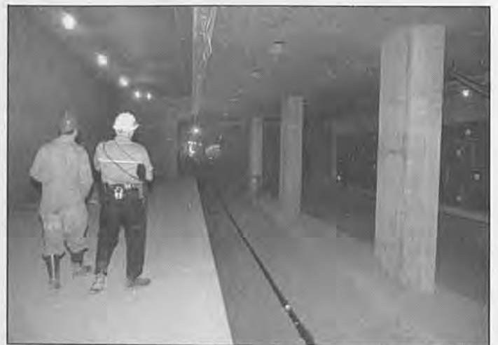
Looking south down the Metro Blue Line alignment, Skeel and Ishkanian appreciate the near completion of the station.
