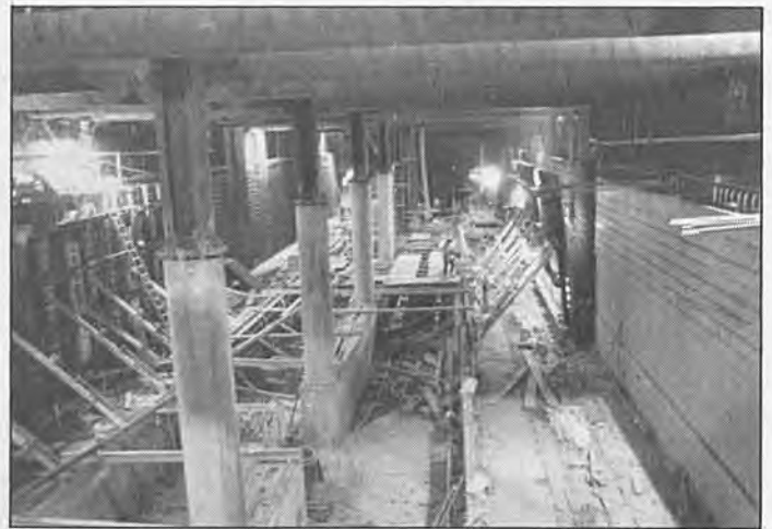
At the 7th and Flower Metro station interface with the Metro Blue Line light rail station, a view from the mezzanine looking down to the Metro Red Line subway level.
