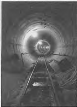
Past the work crew they travel further along the 146 left tunnel alignment.
