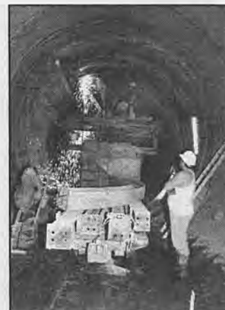
Heading down the 146 alignment, the engineers encounter a work crew setting and welding steel rings for the initial cross-passage construction.
