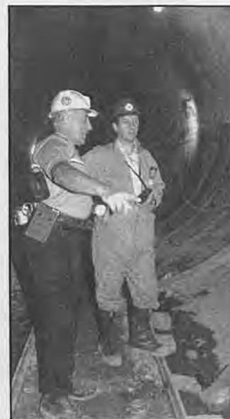
Ishkanian points out the ring steel curved I-beams that are being installed.
