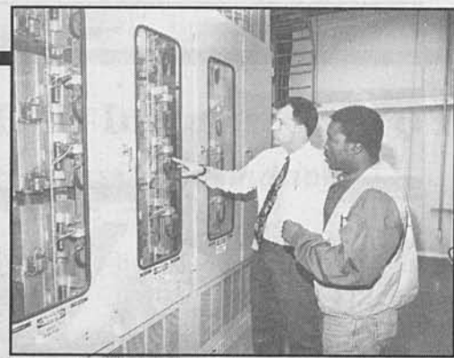
Traction power inspector Francis Mensah and associate engineer Rob Chappell inspect a traction power rectifier, which converts alternating current into direct current.
