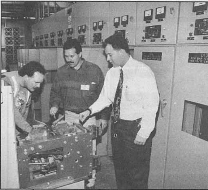
Traction power inspector Louis Perez, traction power supervisor Dave Farley, and associate engineer Rob Chappell inspect the traction power braker in the substation. The electricity comes in from Southern California Edison as alternating current (AC) and is converted to 750 volts of direct current (DC).
