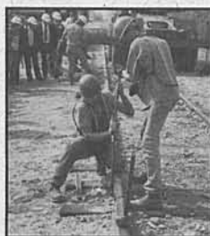
Metrolink workers remove a section of 1899 track during the groundbreaking ceremony of the San Bernardino to Los Angeles commuter rail line.
