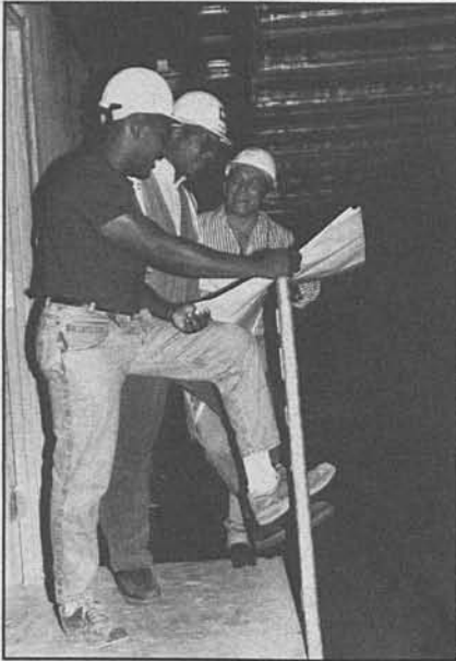
Mikal Sabir, architect inspector; George Flowers, electrical inspector; and Domingo Leon, president of D'Leon Consulting Engineers check architectural finishings at the Metro Center Station / 7th and Flower.
