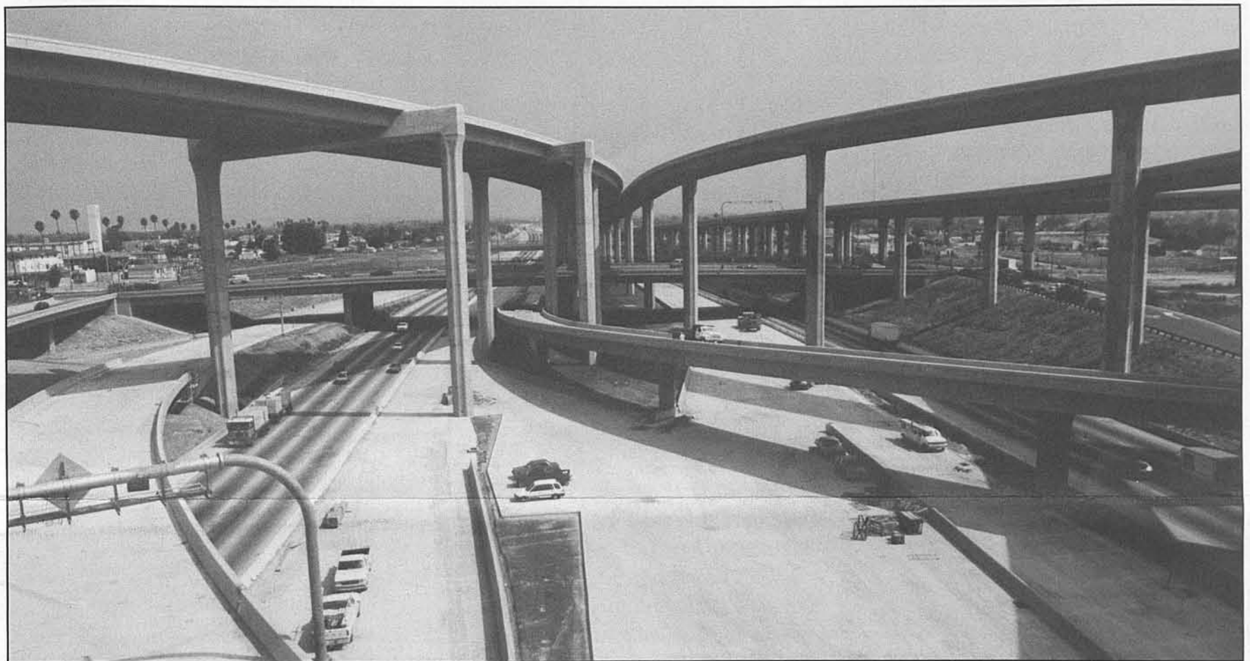
Elevated interchange — A five-level interchange is under construction where the new I-105 meets the Harbor Freeway (I-110). Connecting ramps to be used exclusively by buses, carpools and vanpools are part of the structure, connecting the I-105's HOV lanes to the Harbor Transitway.
