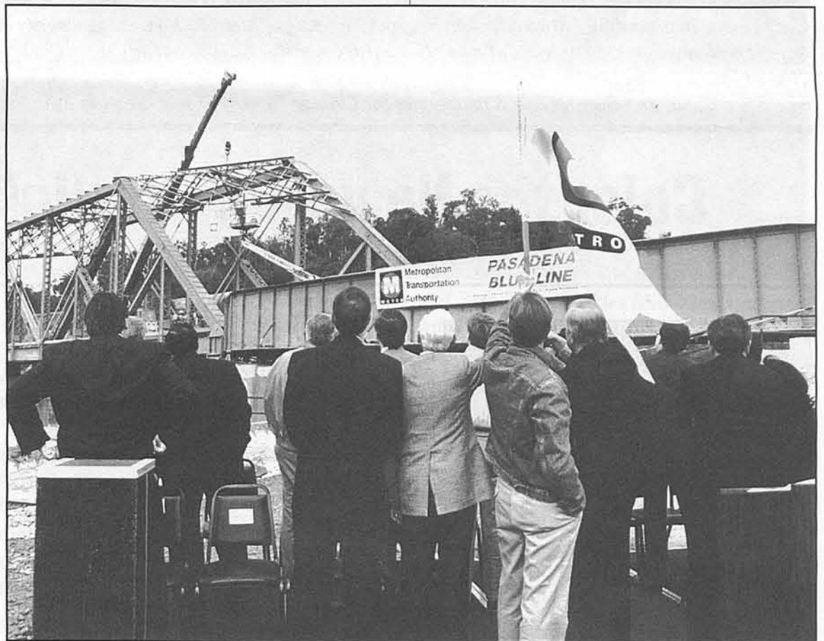
Officials prepare to signal a construction worker in the crane on the bridge to begin work on the Pasadena Blue Line.
