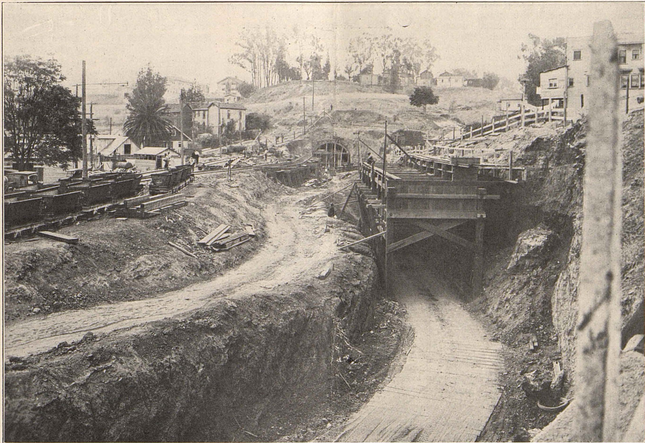
Progress on the new tunnel continues at a good pace. The first drift was started June 13 and another on July 19th. A total of 133 feet of excavation had been removed on July 1st.
