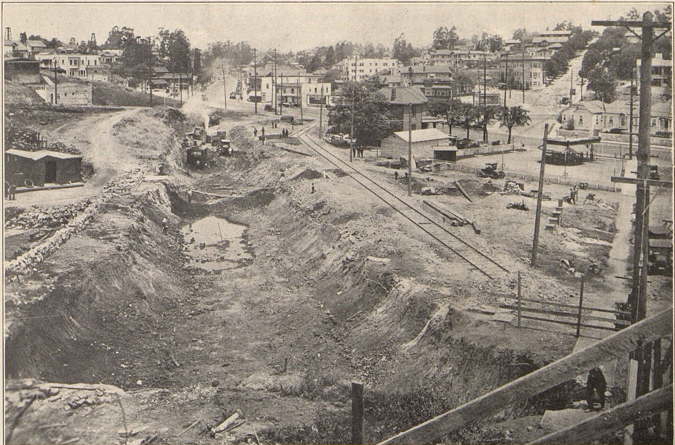
Commendable progress has been made on tunnel project during past month. The immediate foreground is location of western portal where preparations are now being made to start bore. This picture was taken on May 24th.
